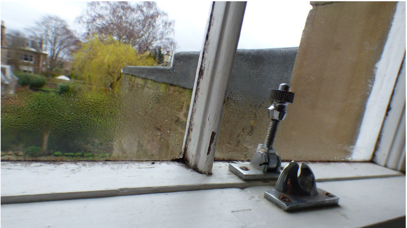
Photograph 22: Showing Window 4 with evidence of a rotten midrail and astragal section. Due to water ingress this section has become beyond repair and requires a replacement sash.
