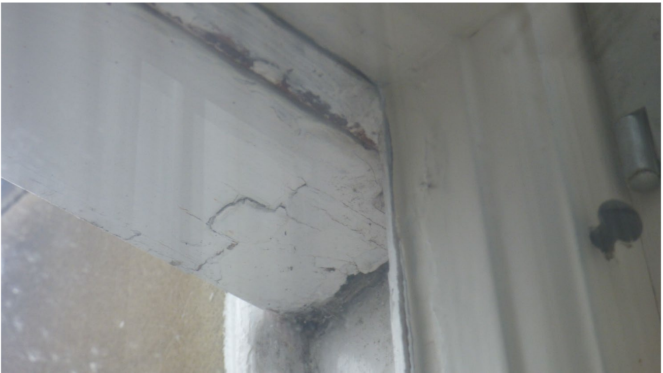
Photograph 11: Showing Window 2 with evidence of a rotten midrail section. Due to water ingress this section has become beyond repair and requires a replacement sash.
