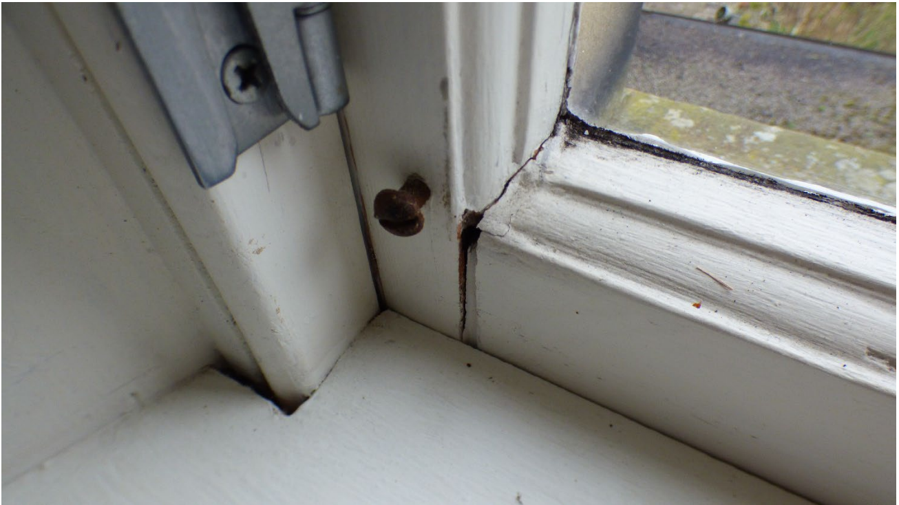
Photograph 16: Showing Window 3 with evidence of a rotten bottom rail section. Due to water ingress the mortice and tenon joint has become rotten and requires a replacement sash.
