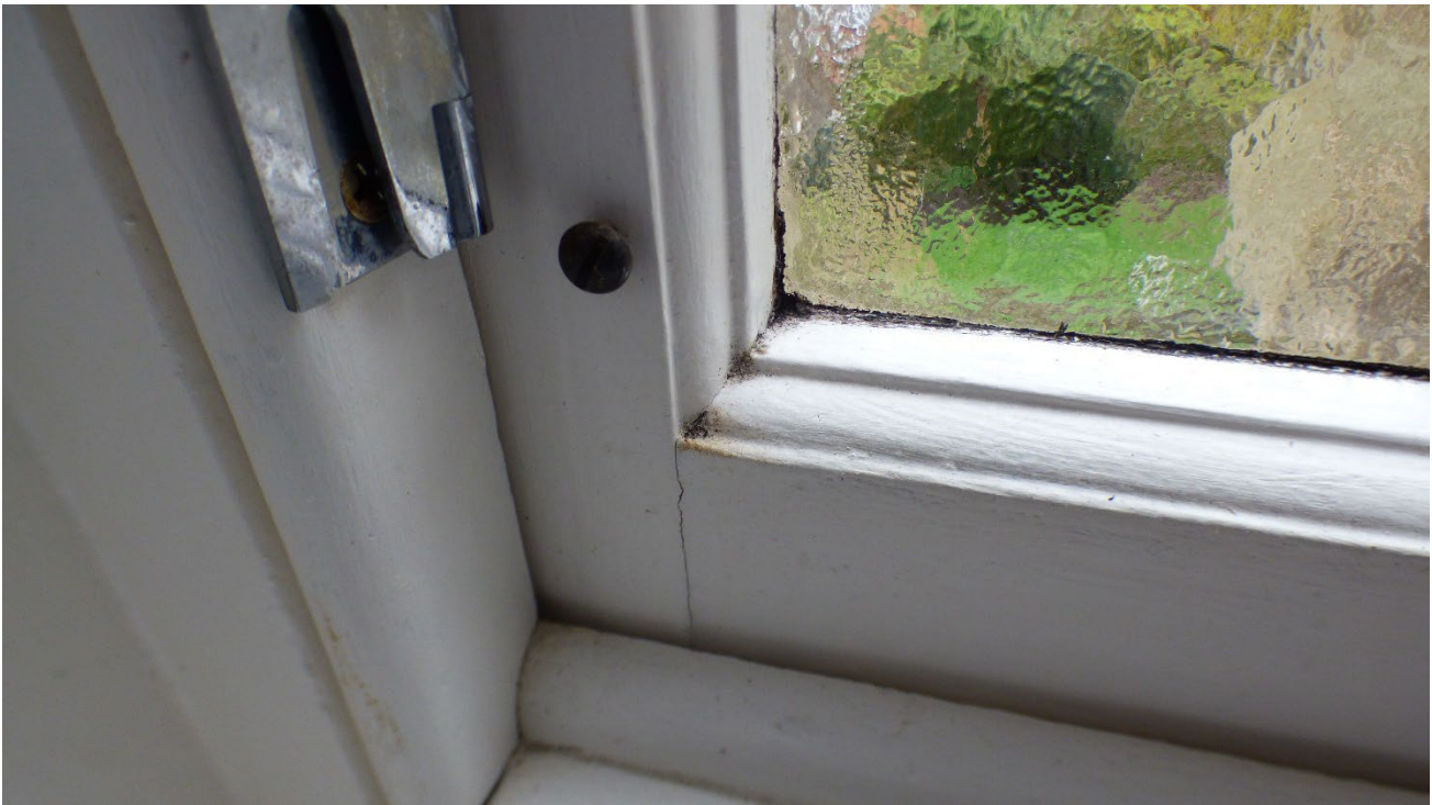
Photograph 21: Showing Window 4 with evidence of a rotten bottom rail section. Due to water ingress this section has become beyond repair and requires a replacement sash.
