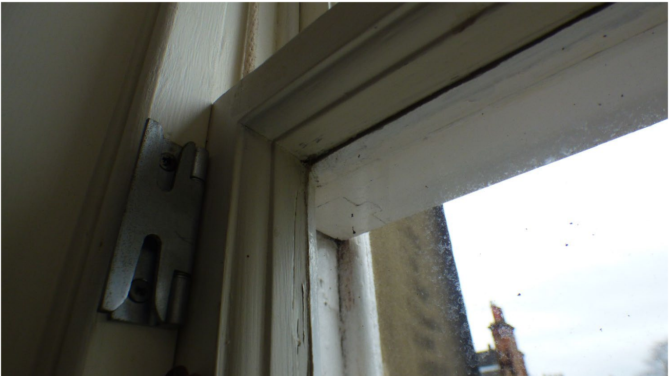
Photograph 18: Showing Window 3 with evidence of a rotten midrail section. Due to water ingress this section has become beyond repair and requires a replacement sash.
