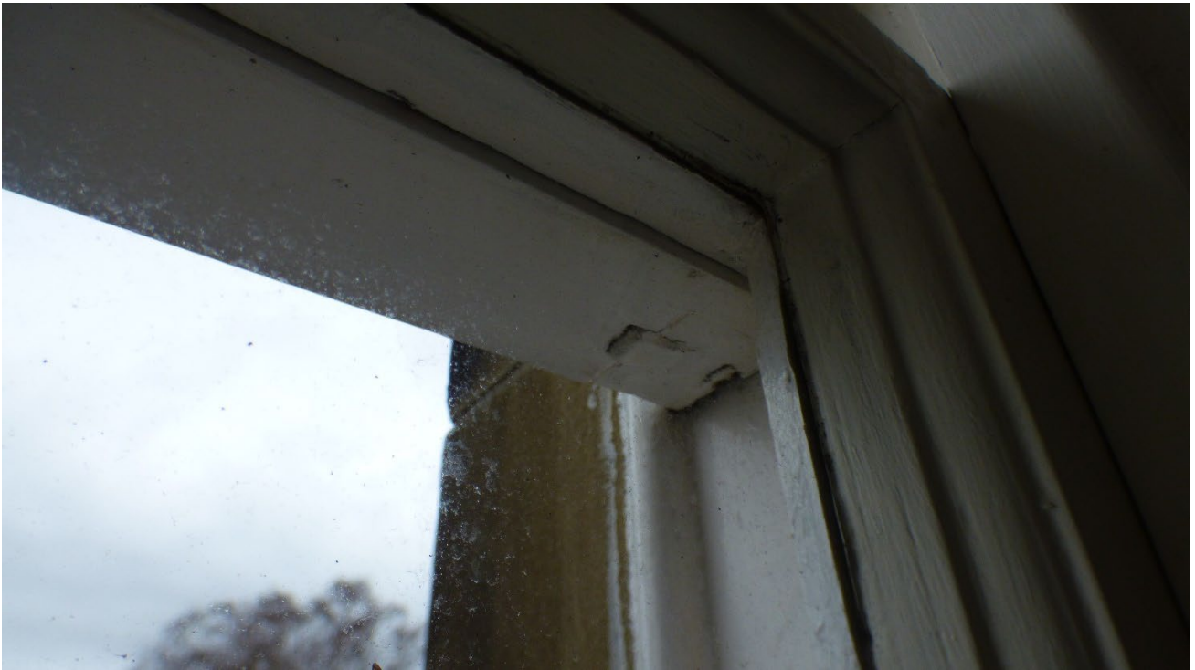
Photograph 17: Showing Window 3 with evidence of a rotten midrail section. Due to water ingress this section has become beyond repair and requires a replacement sash.
