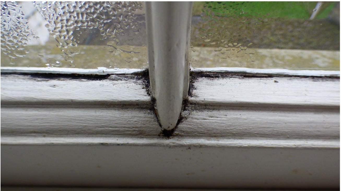
Photograph 15: Showing Window 3 with evidence of a rotten bottom rail and astragal section. Due to water ingress this section has become beyond repair and requires a replacement sash.
