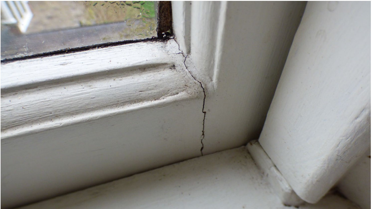
Photograph 14: Showing Window 3 with evidence of a rotten bottom rail section. Due to water ingress this section has become beyond repair and requires a replacement sash.
