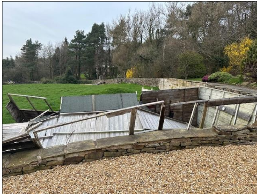
Figure 6: Collapsed Existing Outbuilding.
