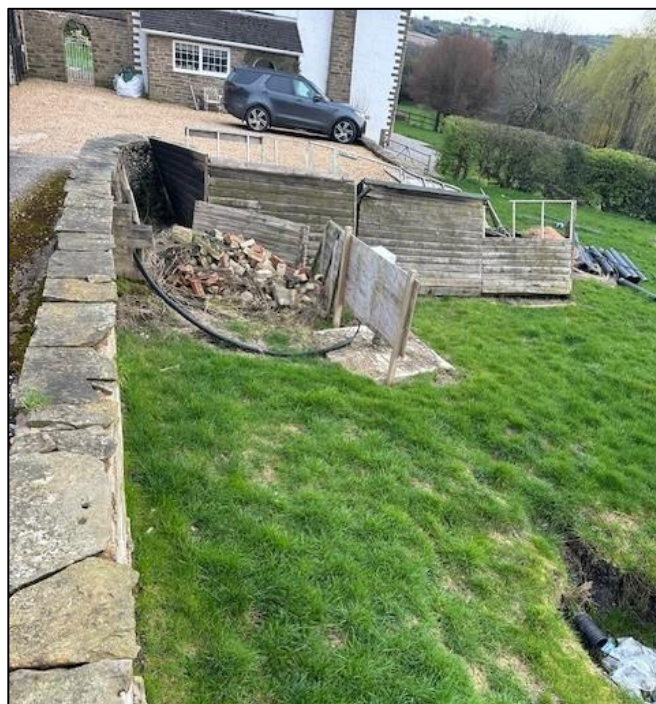
Figure 5: Collapsed Existing Outbuilding.
