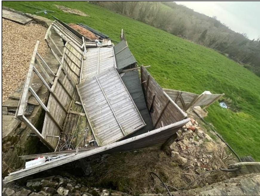
Figure 4: Collapsed Existing Outbuilding.
