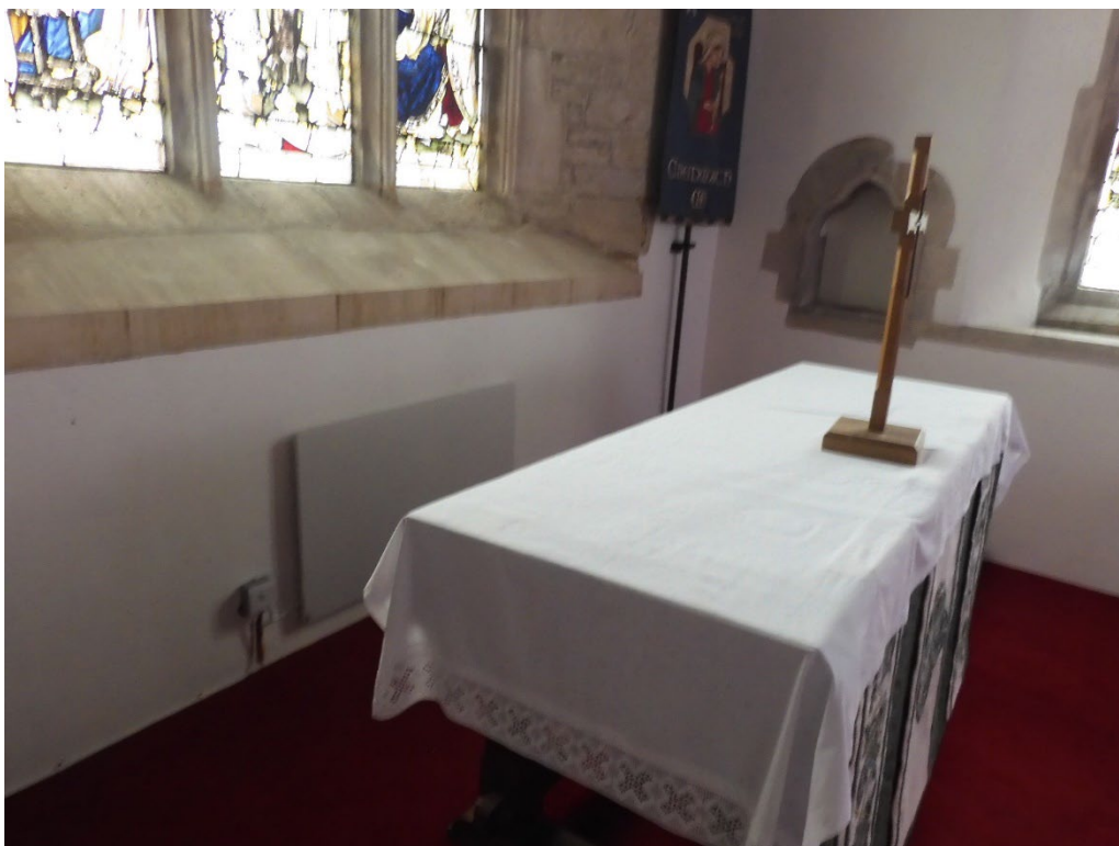
Electric panel heater installed behind an altar.
