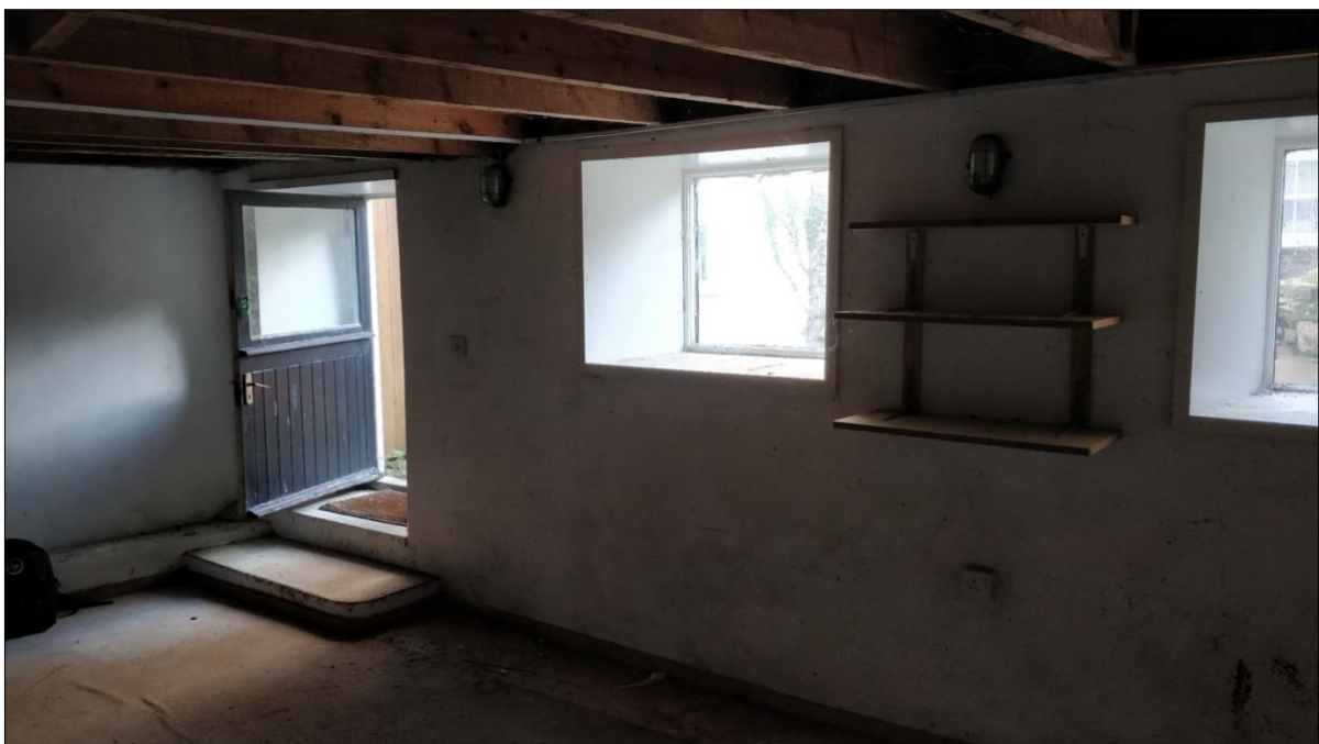
Fig 01 - Internal view showing something of the potential for conversion to a comfortable living space
