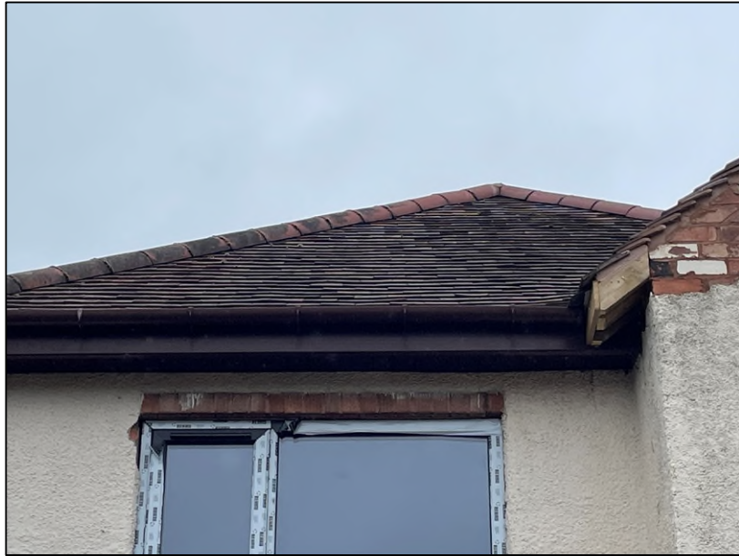
Plate 3: recently repaired gable with open eaves and gaps under tiles. Photograph looking west.
