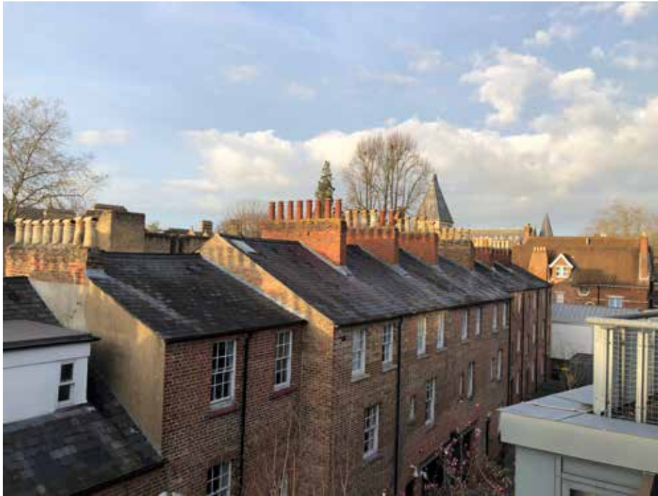
3.16 View of roofs of nos. 1-17 looking NW from top floor balcony of EPA building (DIA)
