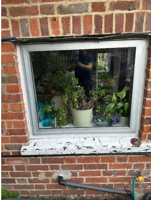
Fig 1.2 Ground Floor Rear Elevation Replacement Existing Concrete cill to be sanded & redecorated
