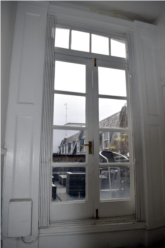
Figure 3.7: Internal view of doors to roof terrace with shutters to either side.
