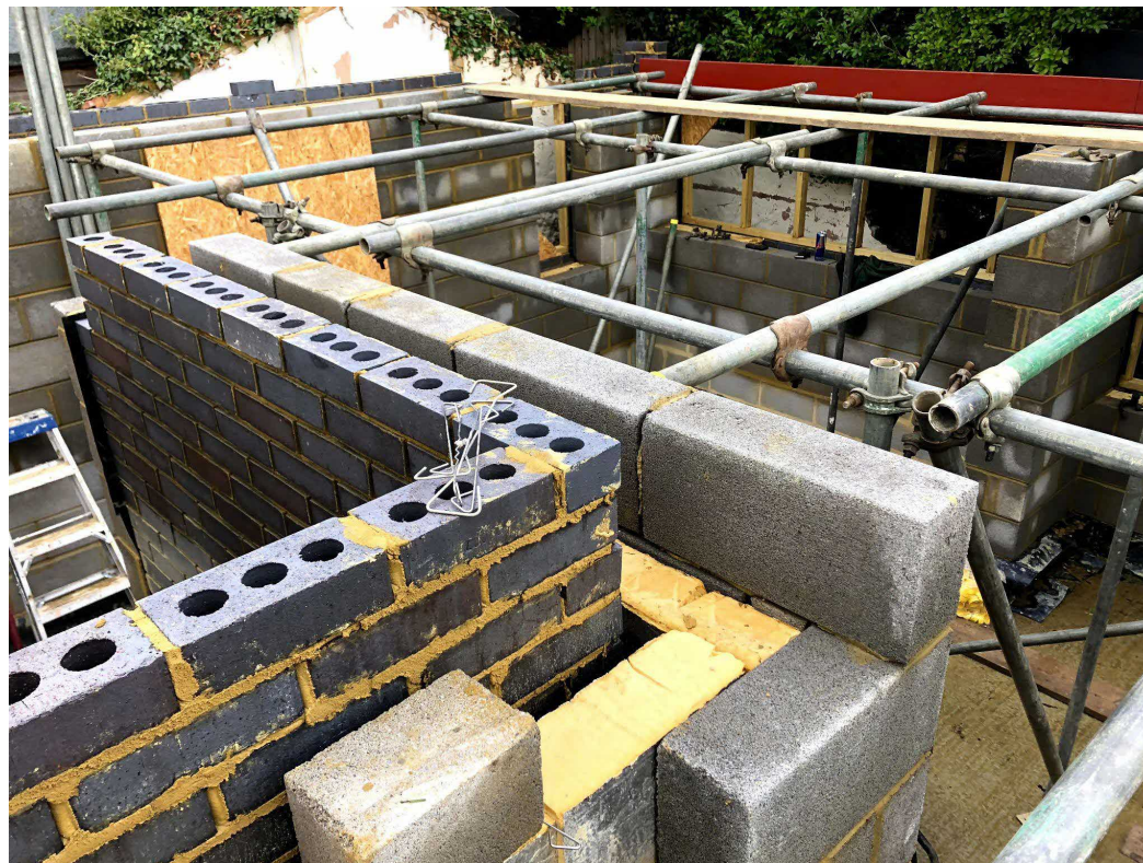
Photograph of the construction of the proposed dwelling showing insulation and extra thick sound deadening concrete blocks in situ
