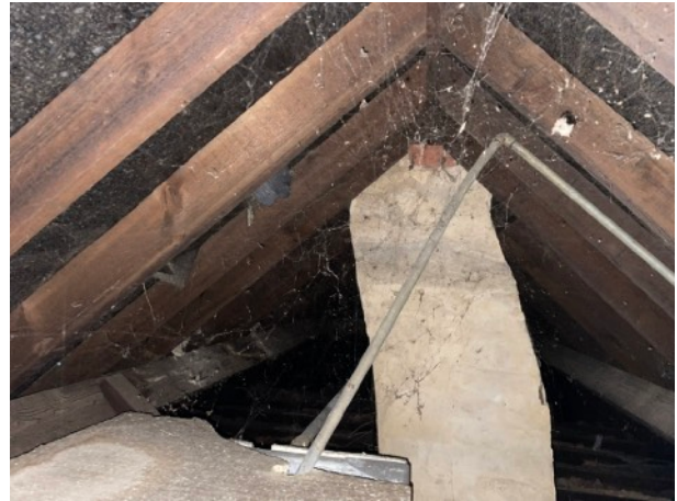
Figure 9. Cobwebs from ridge to floor in loft
