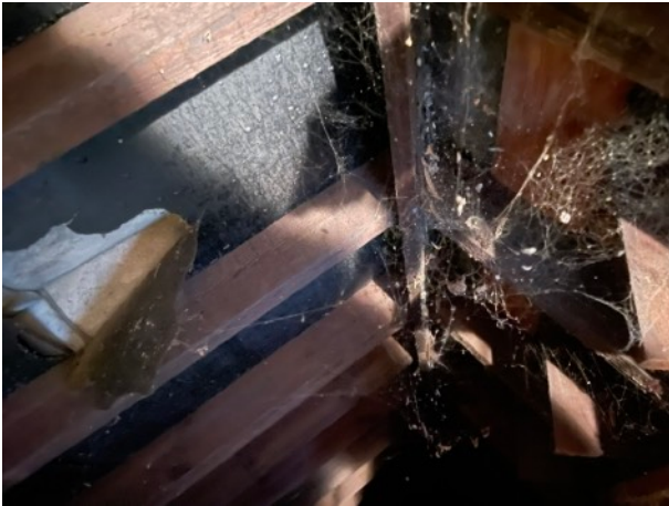
Figure 8. Thick cobwebs at ridge of loft
