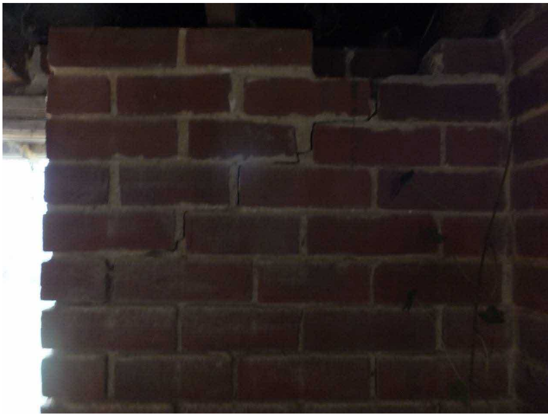
Fig 21 West lean-to –cracking to inner leaf
