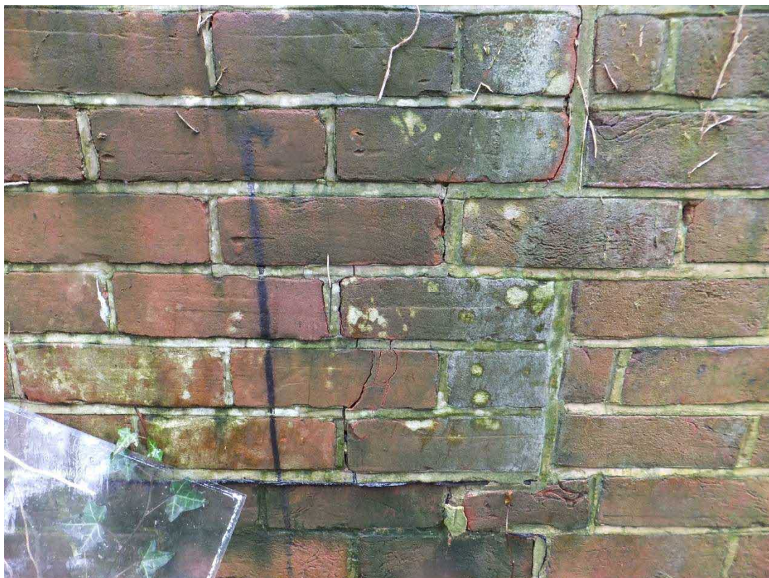
Fig 24 West lean-to –cracking to base of wall
