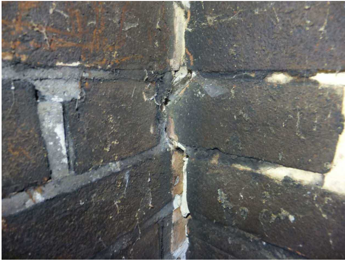
Fig 25 West lean-to –gapping to wall between west lean-to & central section
