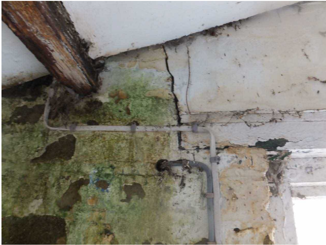
Fig 27 East lean-to –rotten purlin and crack to masonry over lintel
