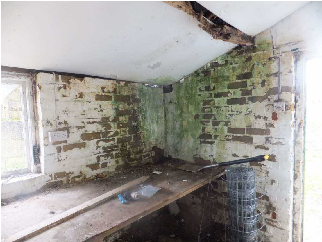
Fig 26 East lean-to –rotten purlin and corner of roof
