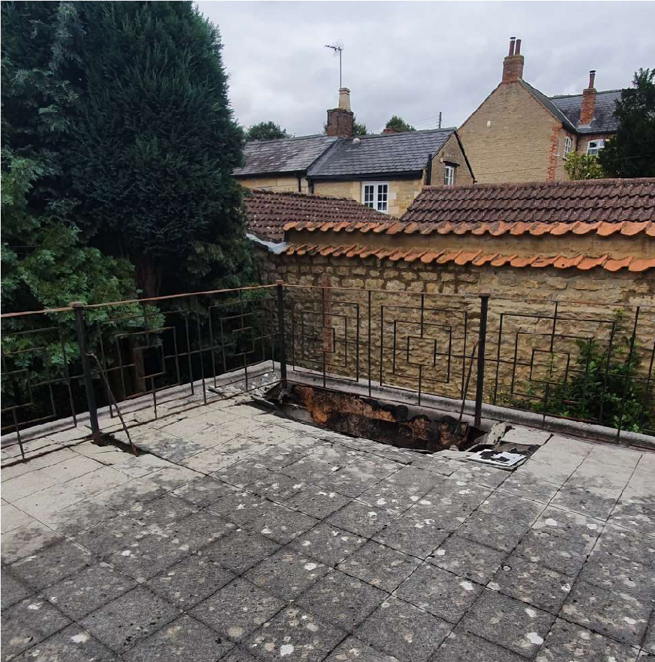
1 - Existing Terrace in unsafe condition
