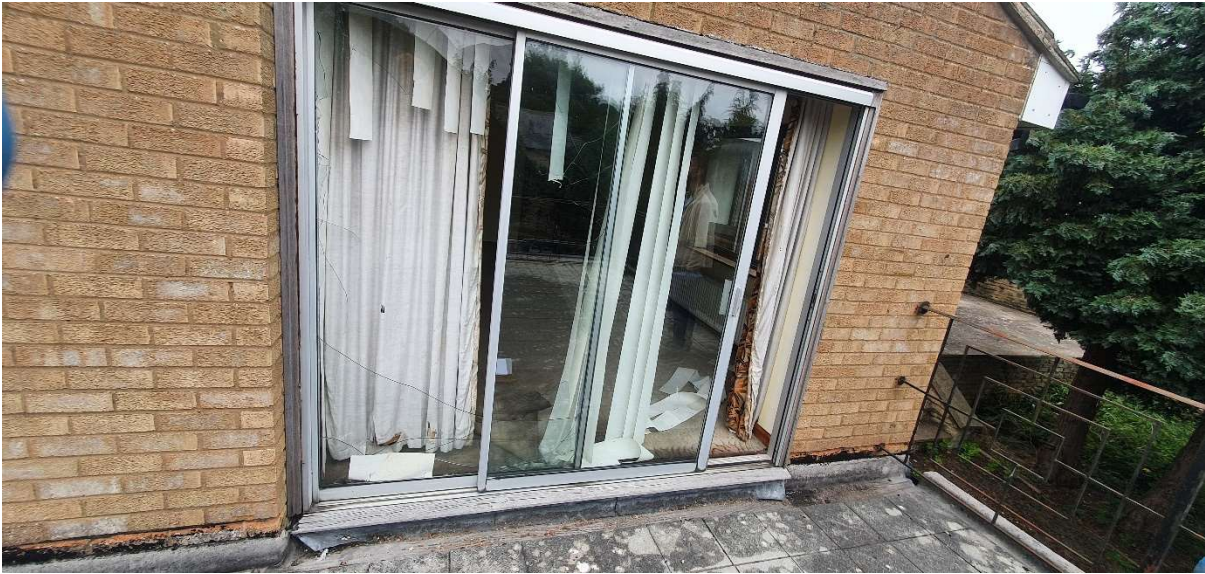
2 - Existing Damaged / Unsafe doors leading to Terrace
