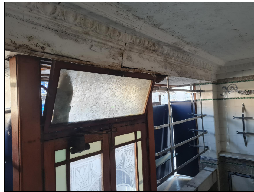
FRONT WALL TO CEILING JUNCTION
