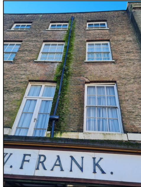
DAMP STAINING AND CRACKING TO FRONT ELEVATION
