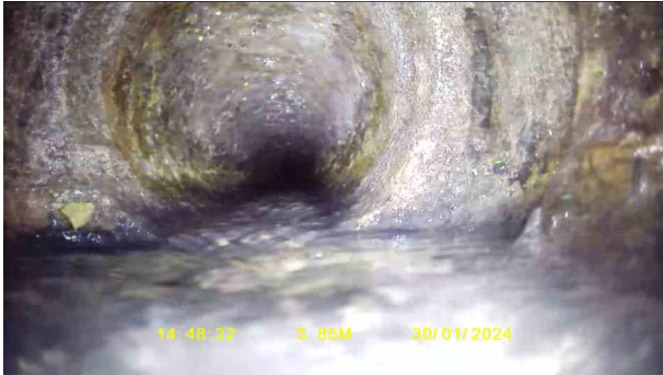
OutfallX_93d762f8-12f5-469f-9b86-62ada8c01128_20240207_144937_656.jpg, 00:02:24, 5.85 m Joint displaced, large
