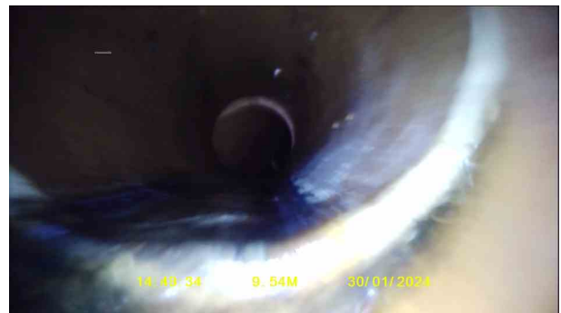
OutfallX_584051a2-19b7-493d-b747-bf505a6b9380_20240207_145213_981.jpg, 00:03:36, 9.54 m Open joint, medium
