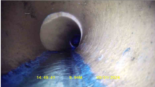
OutfallX_f18fb4c6-9445-4a2d-9f39-cc3abc9c69c4_20240207_145323_863.jpg, 00:03:43, 9.94 m Attached deposits, encrustation from 5 o'clock to 8 o'clock, 10% cross-sectional area loss
