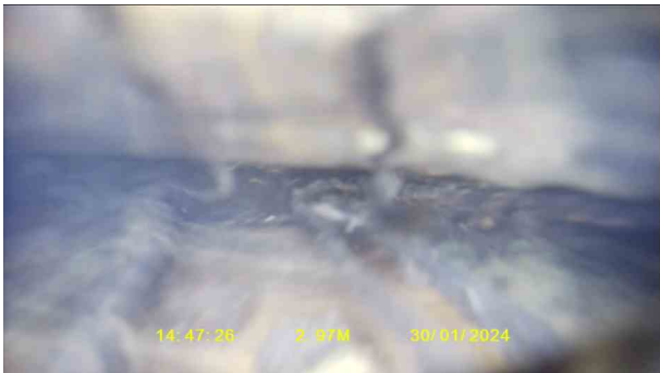
OutfallX_cf4f08d6-c691-42a3-b8a9-d98f67baecac_20240207_144747_279.jpg, 00:01:29, 2.97 m Roots, tap
