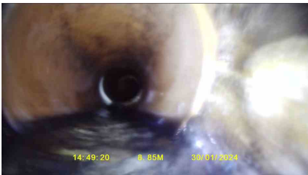
OutfallX_cc939559-63db-41a0-8284-c877ea8fd997_20240207_145139_401.jpg, 00:03:22, 8.85 m Material changes to vitrified clay
