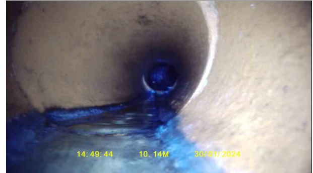
OutfallX_4b33bde6-c209-4661-8d7c-b70650424308_20240207_145338_985.jpg, 00:03:46, 10.14 m Line deviates right
