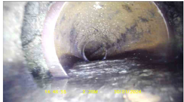
OutfallX_19960c97-f2a0-46d1-bf83-6b4e618f12e7_20240207_144247_636.jpg, 00:00:58, 2.20 m Open joint, large
