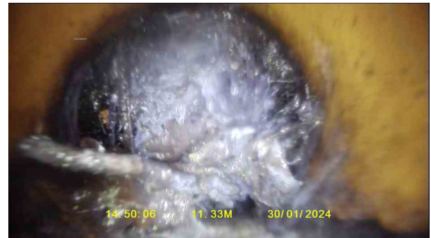
OutfallX_abab79a8-452f-415d-887c-8d16a97969ea_20240207_145517_824.jpg, 00:04:08, 11.33 m Survey abandoned, Line completely blocked
