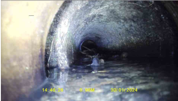
OutfallX_53a77deb-2f96-47fd-89da-481b2703d1a5_20240207_144107_204.jpg, 00:00:31, 0.96 m Open joint, large
