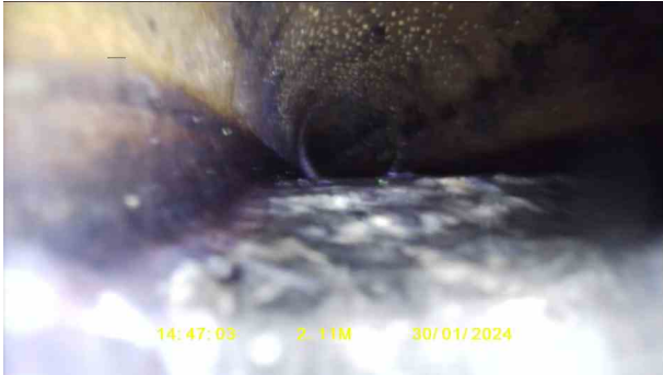
OutfallX_b7b1b047-8d08-4d7e-bbb0-a86f977c5ef5_20240207_144325_629.jpg, 00:01:06, 2.21 m Settled deposits, coarse, 15% cross-sectional area loss
