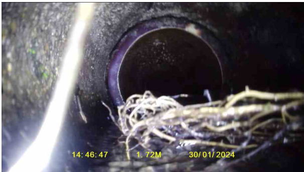
OutfallX_1bfe1504-e6ec-4b6d-a041-c26e970ff7de_20240207_144209_986.jpg, 00:00:49, 1.72 m Roots, mass, 15% cross-sectional area loss
