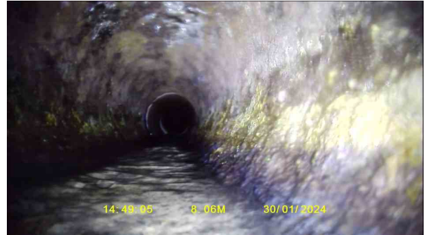
OutfallX_839c829b-a3ec-4679-a72c-4b693fa7b2f7_20240207_145047_743.jpg, 00:03:07, 8.06 m Attached deposits, encrustation from 4 o'clock to 8 o'clock, 15% cross-sectional area loss
