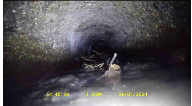
OutfallX_30ab77ca-0060-4b10-8d18-56899995f9c8_20240207_144134_623.jpg, 00:00:40, 1.24 m Settled deposits, coarse, 15% cross-sectional area loss
