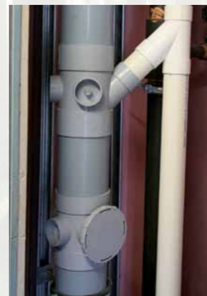
Secondary ventilated stack
