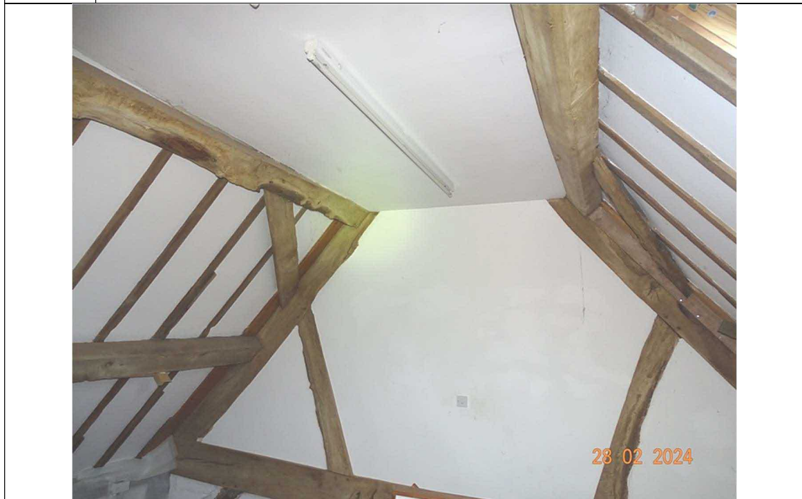
Fig 12. Describing vaulted ceiling which runs full length of building above other first floor compartments.
