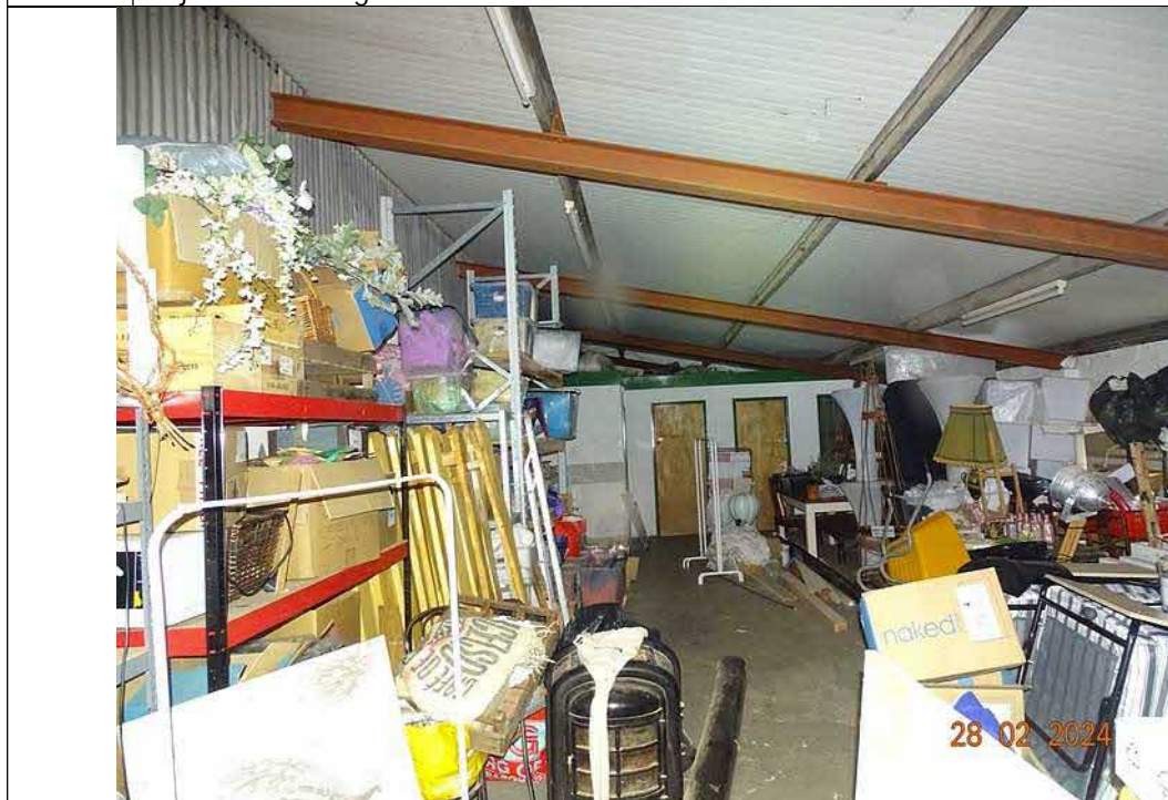
Fig 8. Looking along inside of rear extension, describing roof construction. Doors at far end are into storage rooms. No access was available on the day of the survey. Note open space above doors used for storage, so room deemed highly unlikely to be used by roosting bats.
