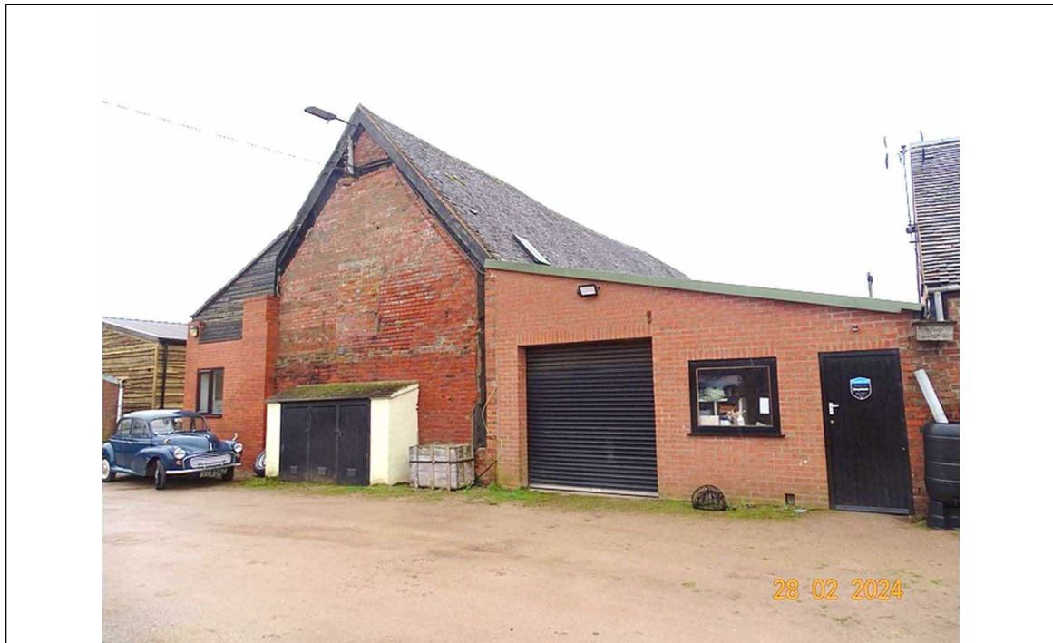
Fig 7. Describing northerly lean too extension at rear of building and its junction with adjacent building.
