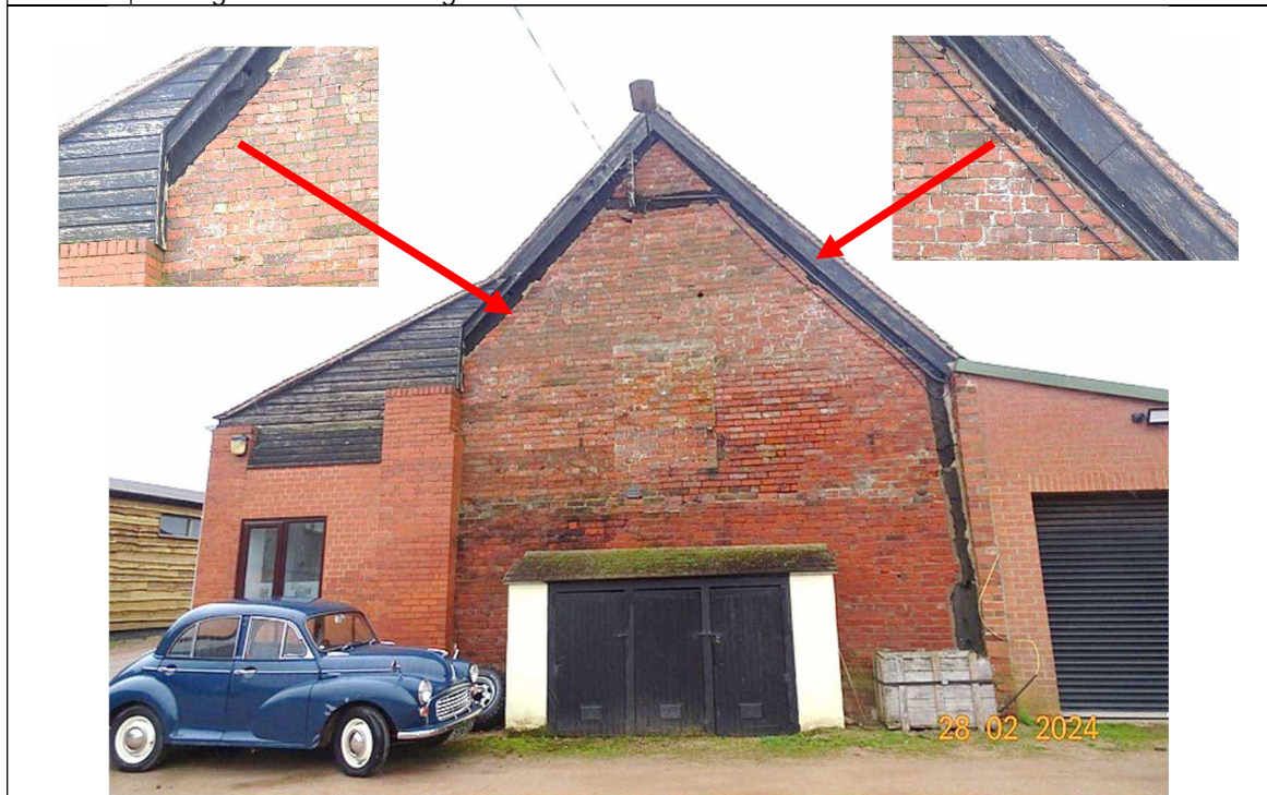
Fig 6. Describing east gable. Inset photos show gaps at wall top / timber wall plate junctions which could give access for roosting bats.
