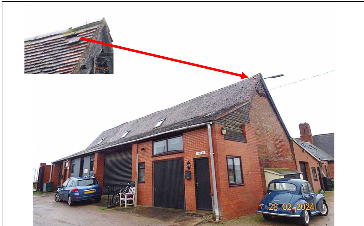
Fig 5. Describing building from southeast. Inset photo of dislodged tile with potential access to ridge tiles for roosting bats.
