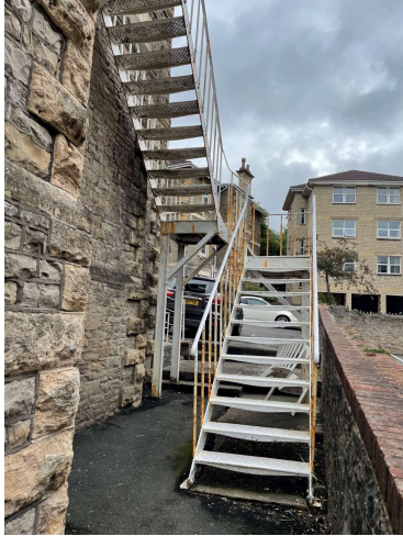
Dilapidated external staircase
