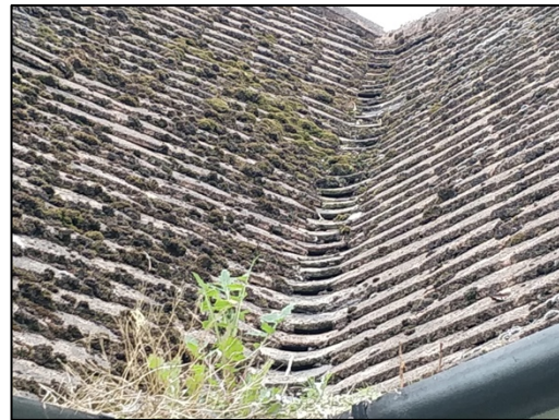
Figure 6 – gaps under the corner hip tiles
