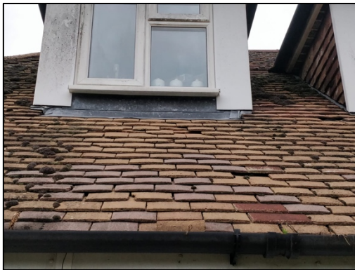
Figure 5 – gaps under and slipped roof tiles
