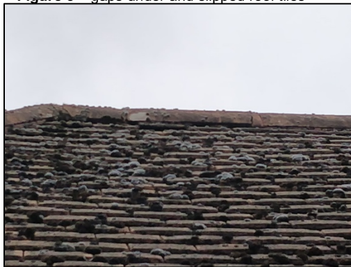
Figure 7 – missing mortar under the ridge tiles
