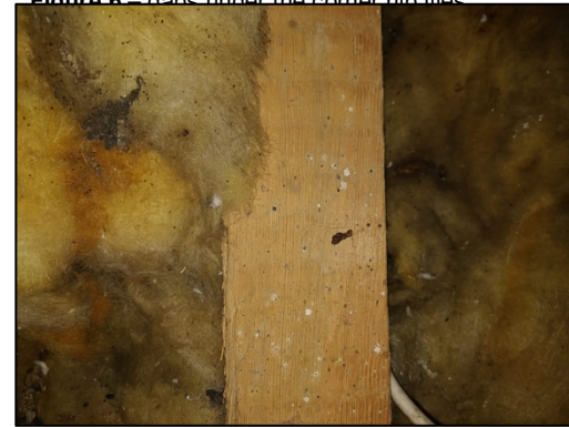
Figure 8 – long-eared type bat dropping inside the void
