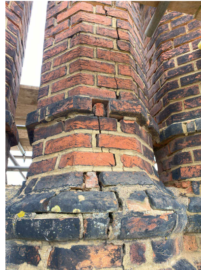
Flue stack 5A showing crack
