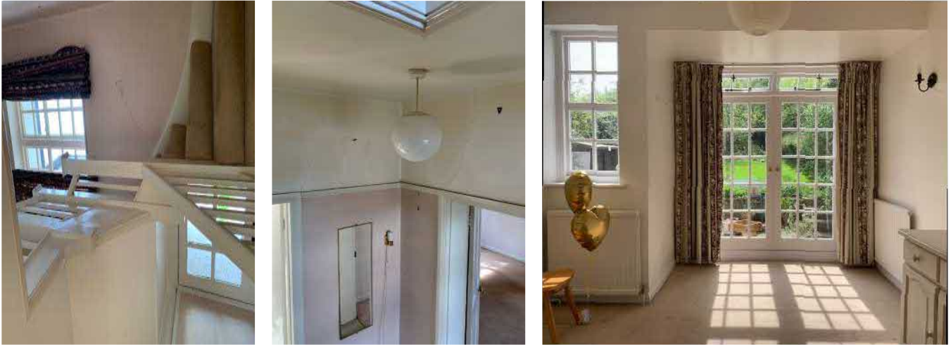
Interior views showing the existing staircase, hallway and dining room. Interior and exterior walls show signs of movement.
