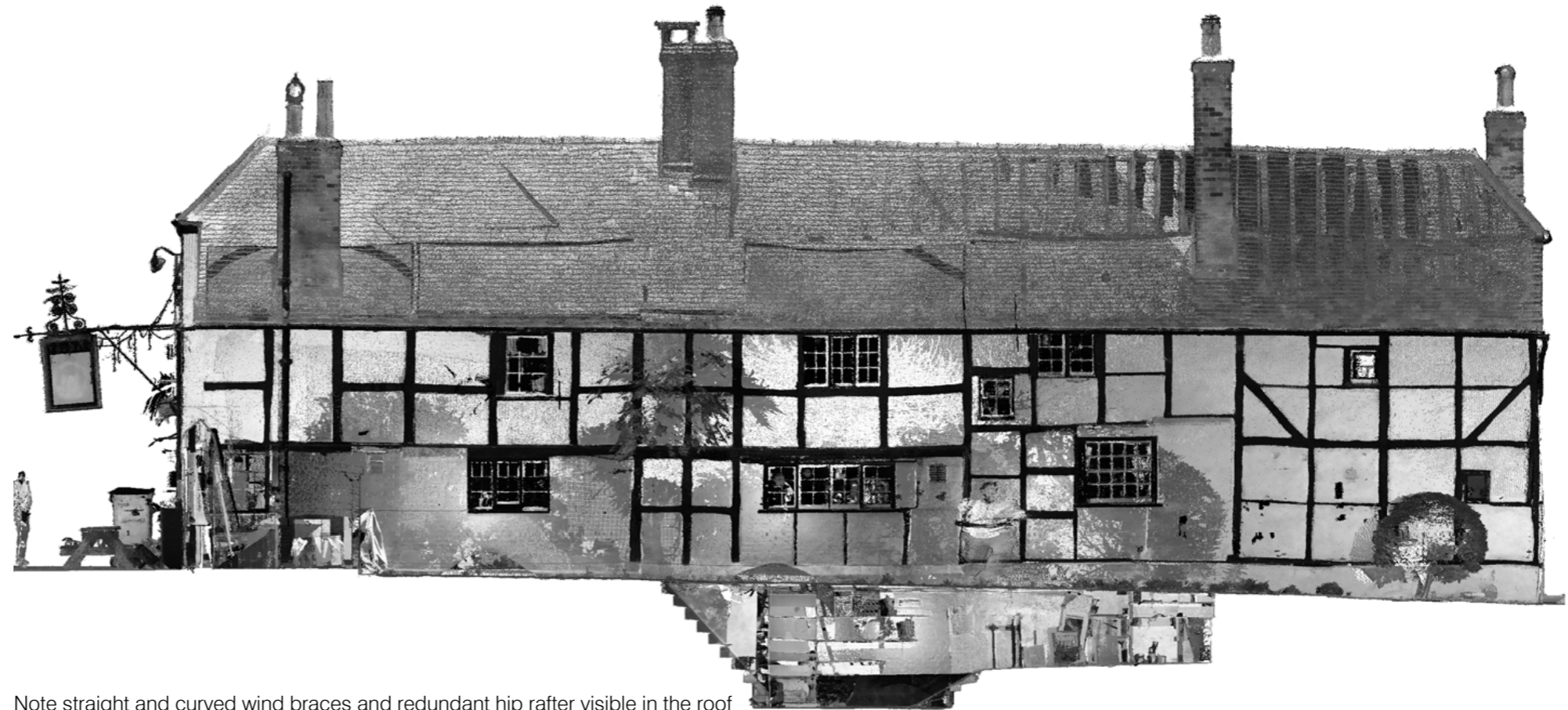
Note straight and curved wind braces and redundant hip rafter visible in the roof
