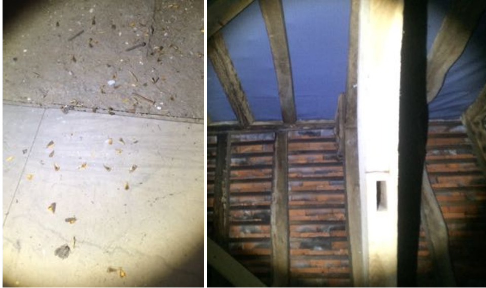
Figure 3- Feeding remains recorded underneath ridge and beam features towards the western elevation, prior to the survey conducted on 27th August 2021.
