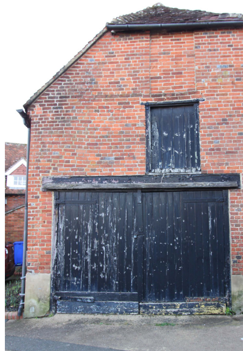
Delapidated joinery openings
