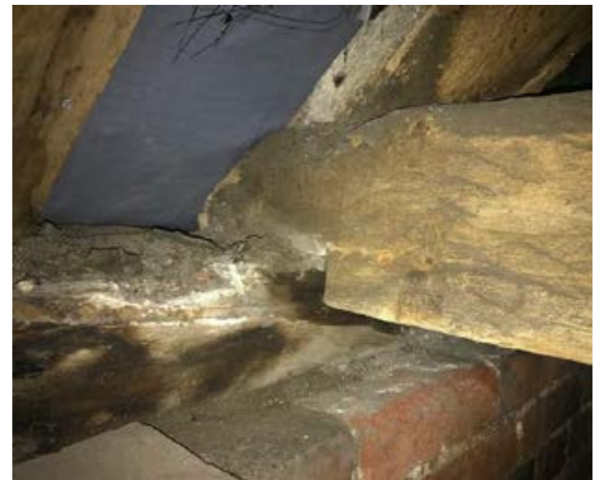
Above: Handmade clay peg tiles are hung using ferrous roofing nails which have corroded Note size of wall plate and pegged half-lap scarf joint supported on solid brick wall Below: Decay to joint between tie beam and wall plate. Dovetail missing from wall plate.
