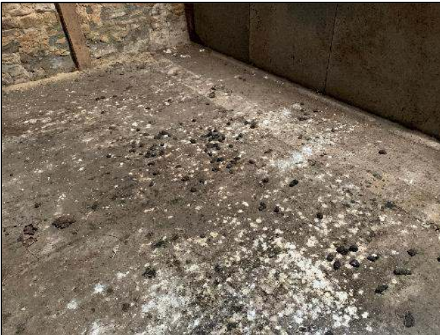
Photograph 15 Building Reference 8, internal – large accumulation of barn owl pellets
