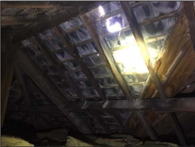
Photograph 7 Loft void of Building Reference 3, showing holes in roof.
