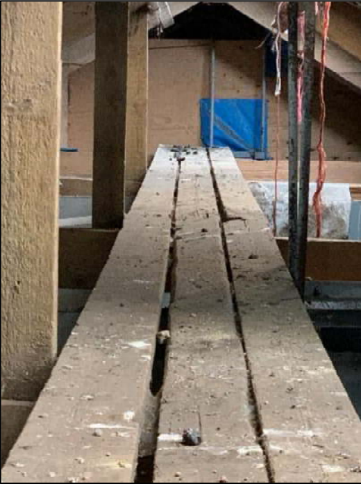
Photograph 17 Building Reference 8, internal – barn owl pellets along upper walkway of grain store.
