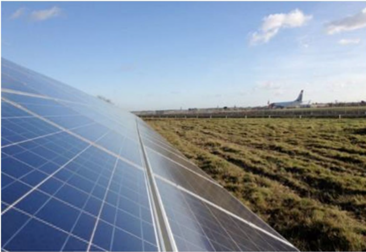
Figure 2: Solar Array next to Gatwick Runway (Business Green, 2013 10 )
