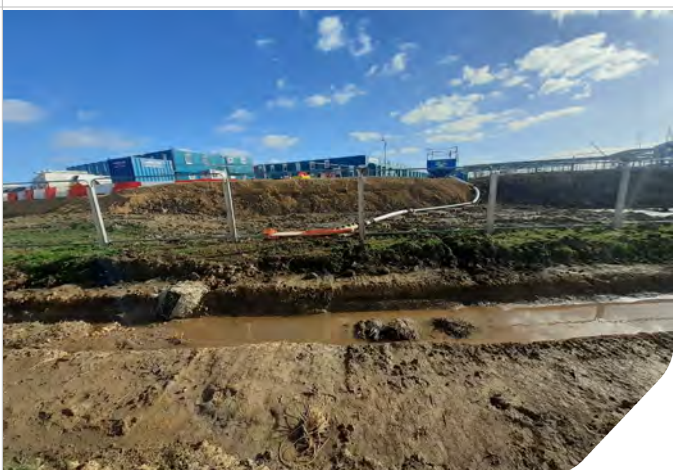
Photo 17: Drainage from Plot 1
