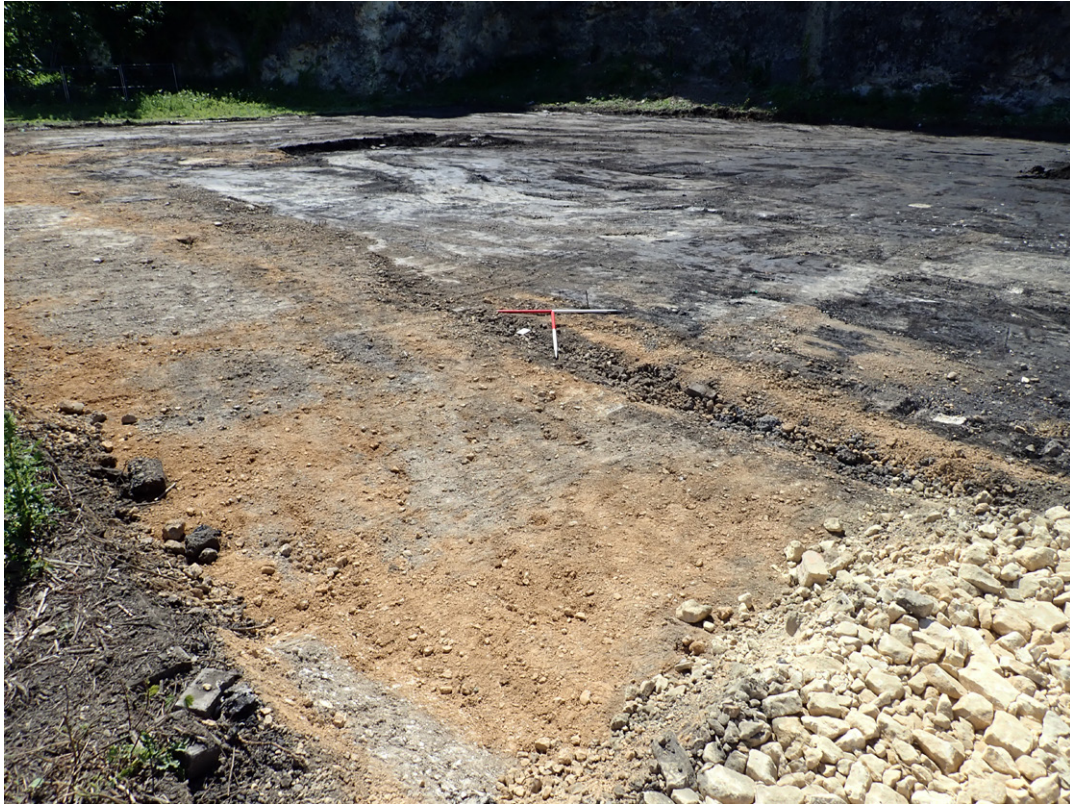
Fig. 3.11: Excavation to required depth in eastern general working platform, Area 2, facing south-east
