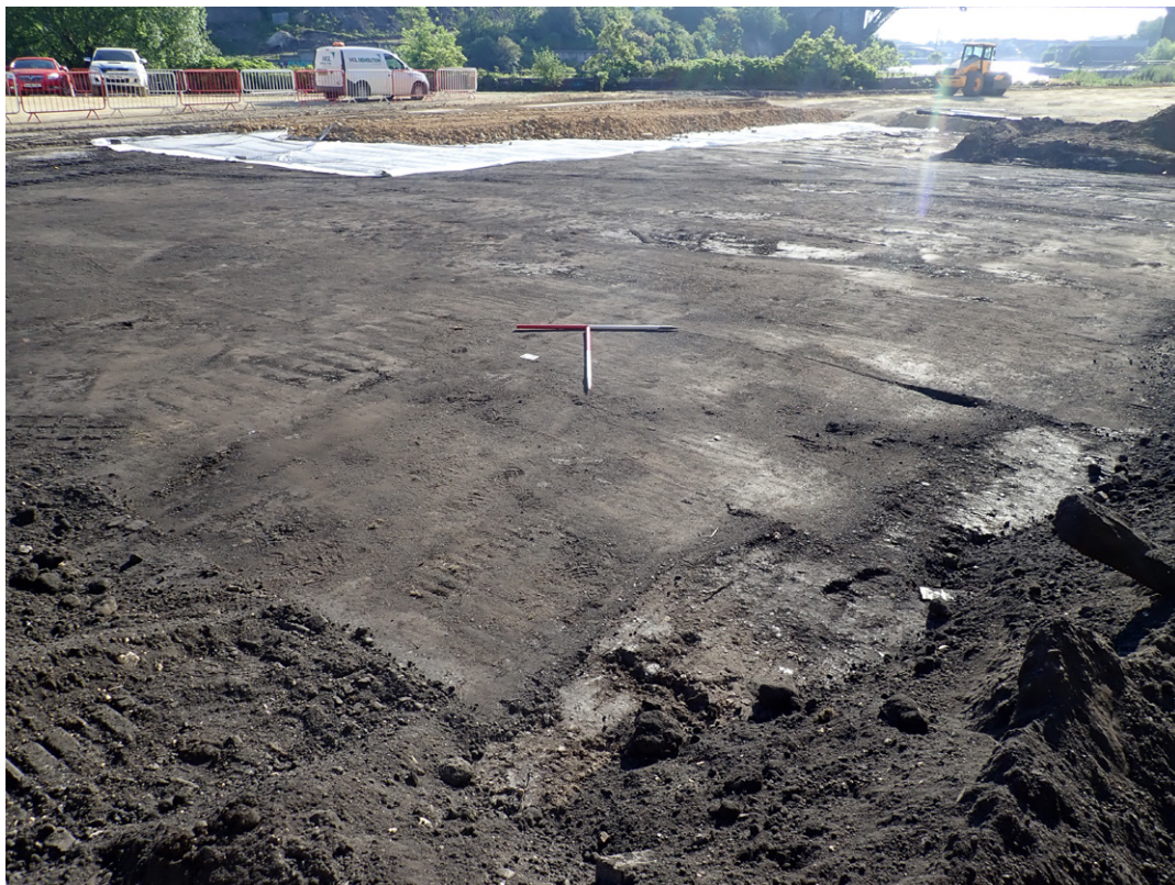
Fig. 3.12: Excavation to required depth in western general working platform, Area 2, facing north-east
