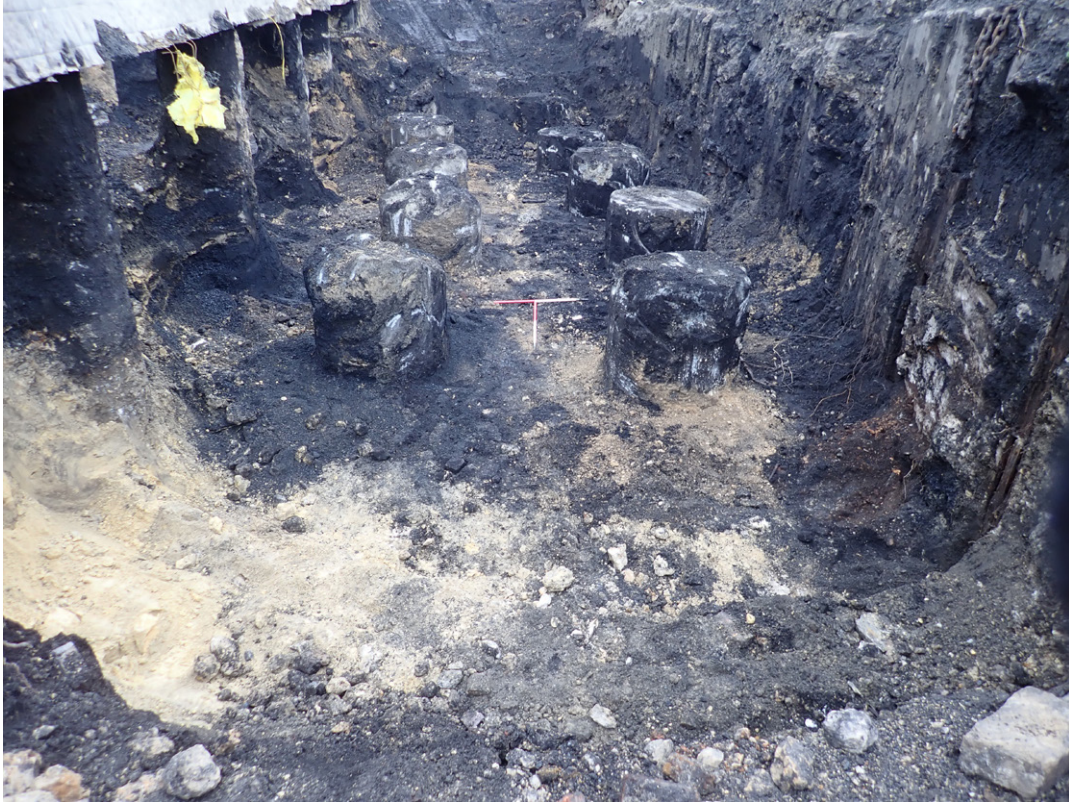
Fig. 3.39: South Pier pit excavation, approximately 5m down from ground level, facing west
