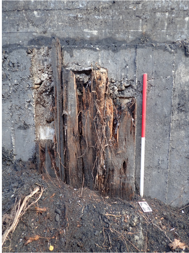
Fig. 3.59: Wooden sleepers against the retaining wall showing marks in reinforcement concrete, north-western access ramp to South Pier pit
