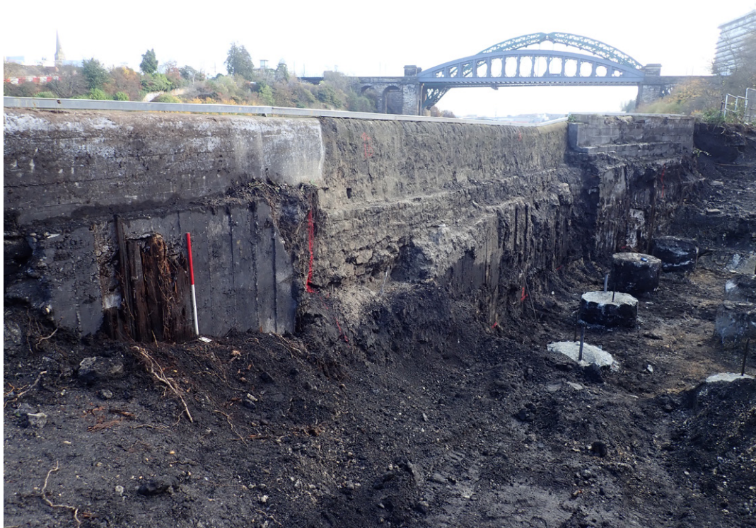
Fig. 3.60: Location of wooden sleepers against the reinforcement of the retaining wall, north-western access ramp to South Pier pit
