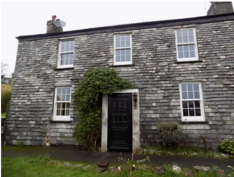
Pic 1. The primary early C19 south elevation symmetrical frontage and slate hung.
