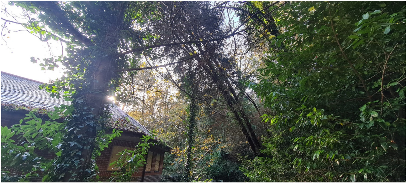
G26 Chinese Juniper in poor condition and leaning over octagonal building within site. This tree should be felled.
