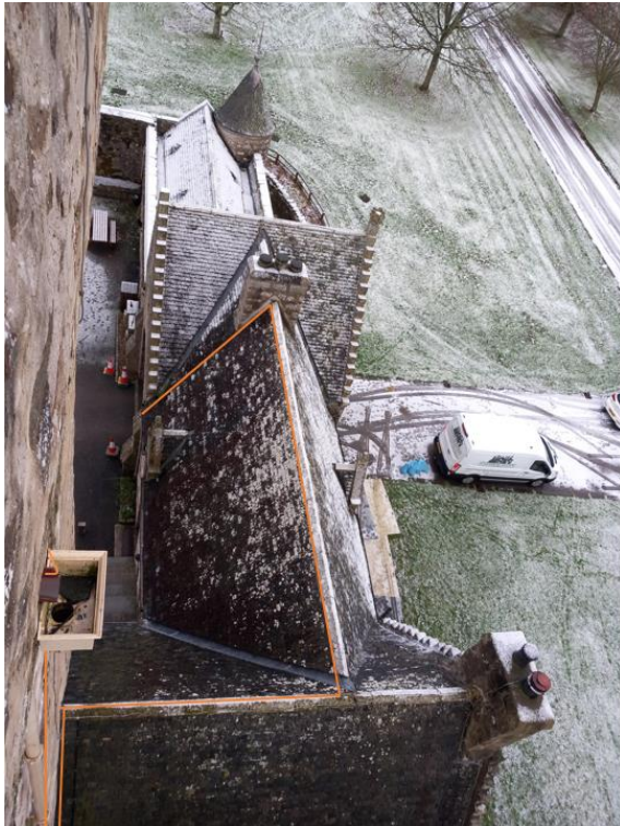
Fig. 21 Line of proposed cabling down from hopper, along ridgeline into Tower Store.
