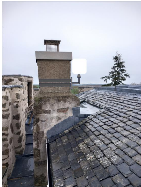
Fig.5 Photomontage (not to scale) of chimney with Starlink receiver on east side of chimney facing north
