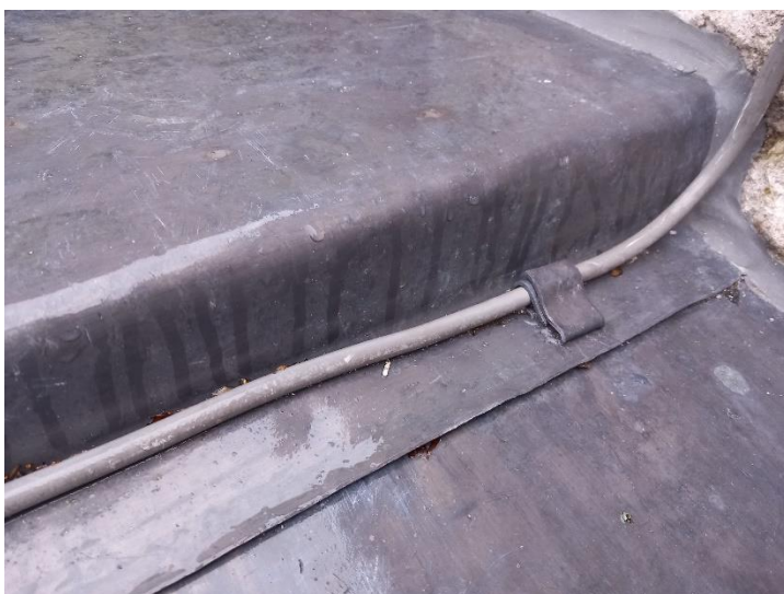
Fig. 23 Example of existing lead clip holding cable in place across lead covered walkway
