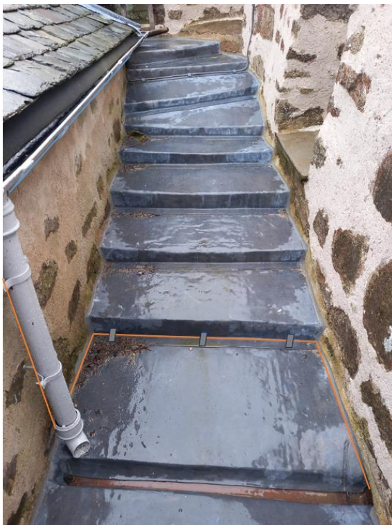
Fig.19 Cable route shown in orange. From cap house gutter across walkway to downpipe
