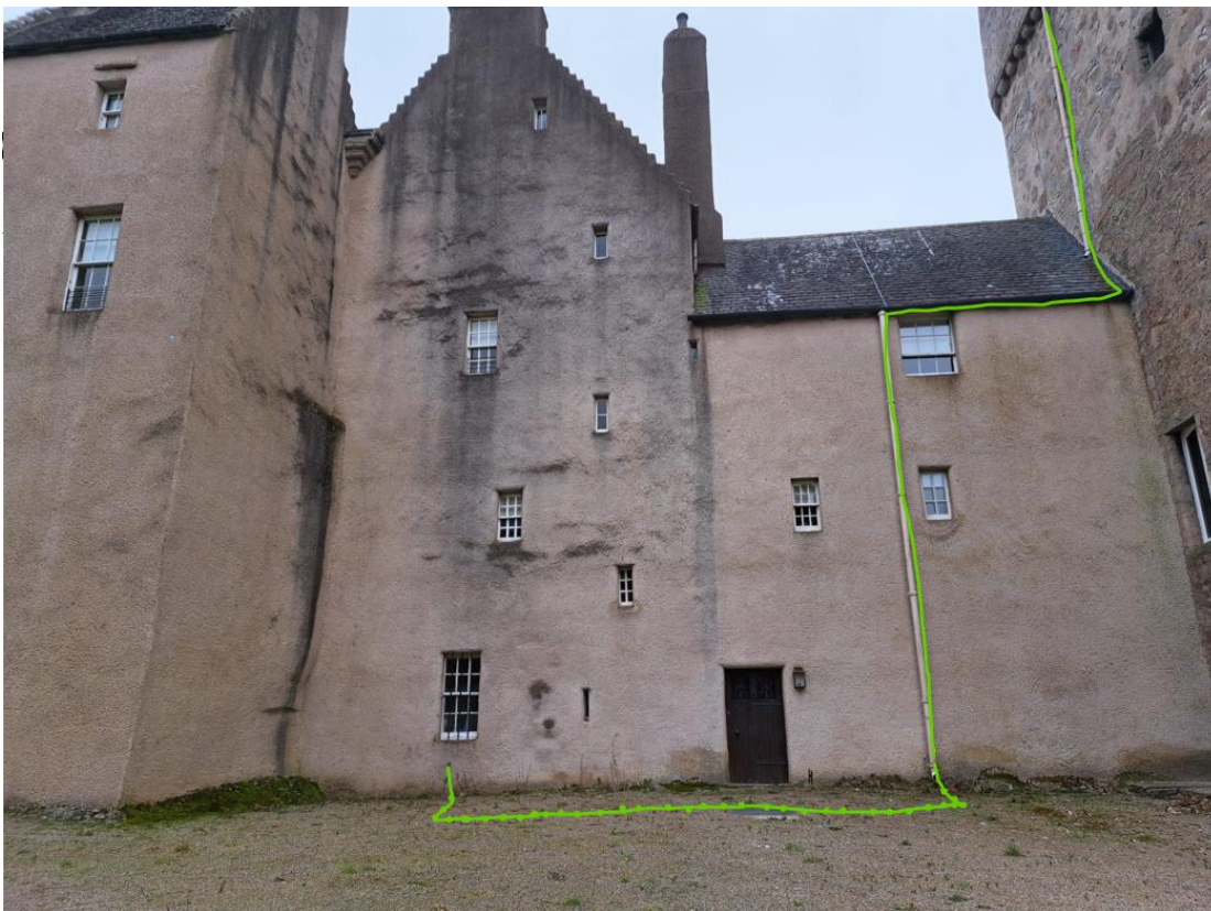
Fig. 18 Dotted section of proposed trenching route to avoid doorstep and drain cover
