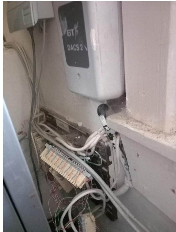
Fig.17 Internal office area adjacent to window for equipment cabinet.
