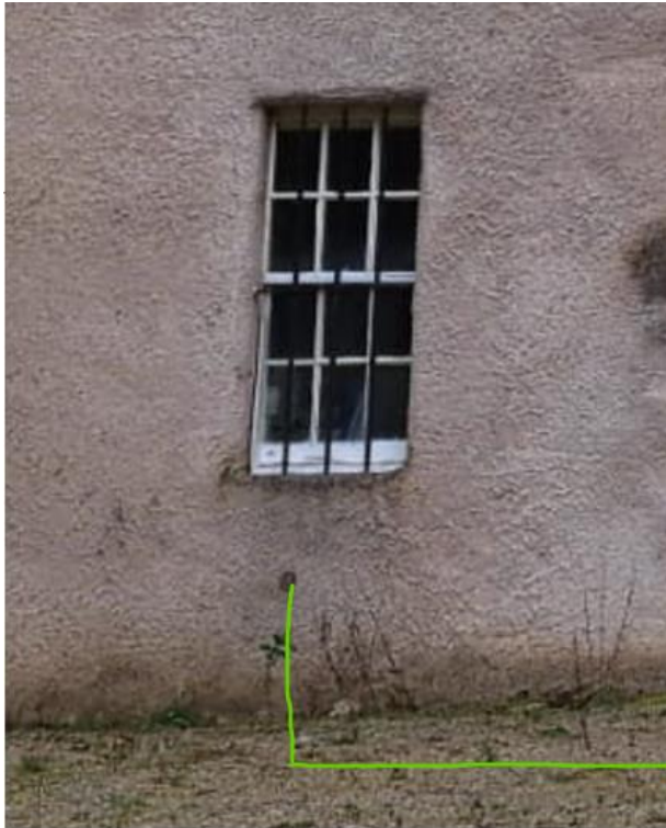
Fig. 16 Reopen existing filled in hole through wall under window into NTS office
