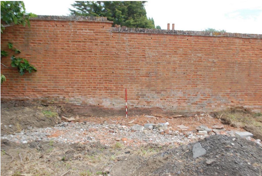
Plate 12 Internal north-west facing wall and location of proposed new access, looking south-east scale 1m
