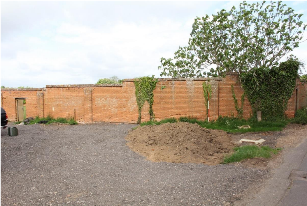
Plate 5 External south-east wall (location of proposed new access), looking north-west. Scale 2m
