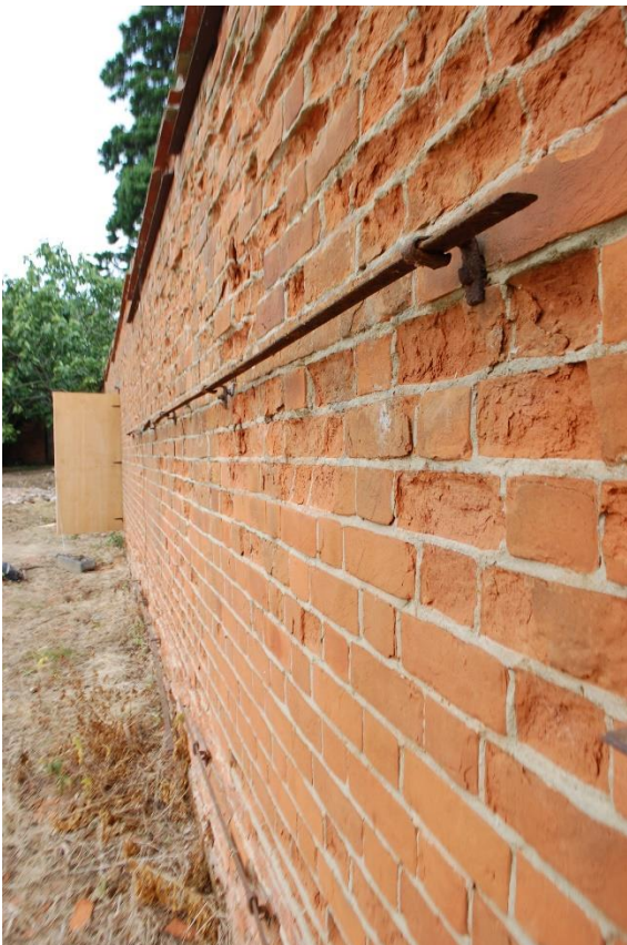
Plate 14 Detail of metal fixings and rails for espalier trees and shrubs, looking north-east
