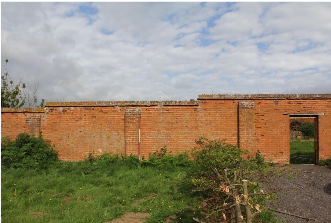
Plate 4 External south-east wall, shallow buttress, and side entrance, looking north-west. Scale 2m
