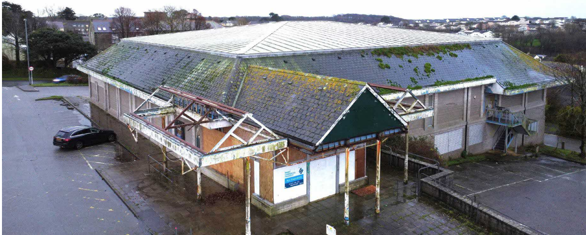
Aerial photo of poor condition tiled and metal roofs to be cleaned and refurbished
