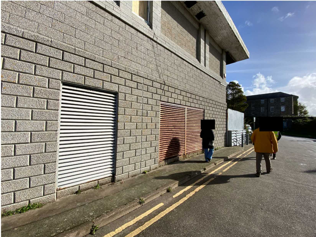
South-West elevation: Boarded up windows and rusted metal louvre panels
