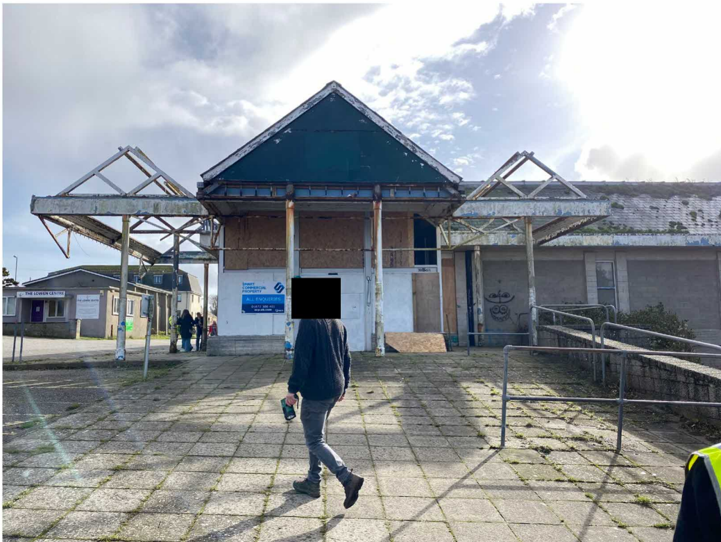
Existing poor condition main entrance and dilapidated canopy steelwork
