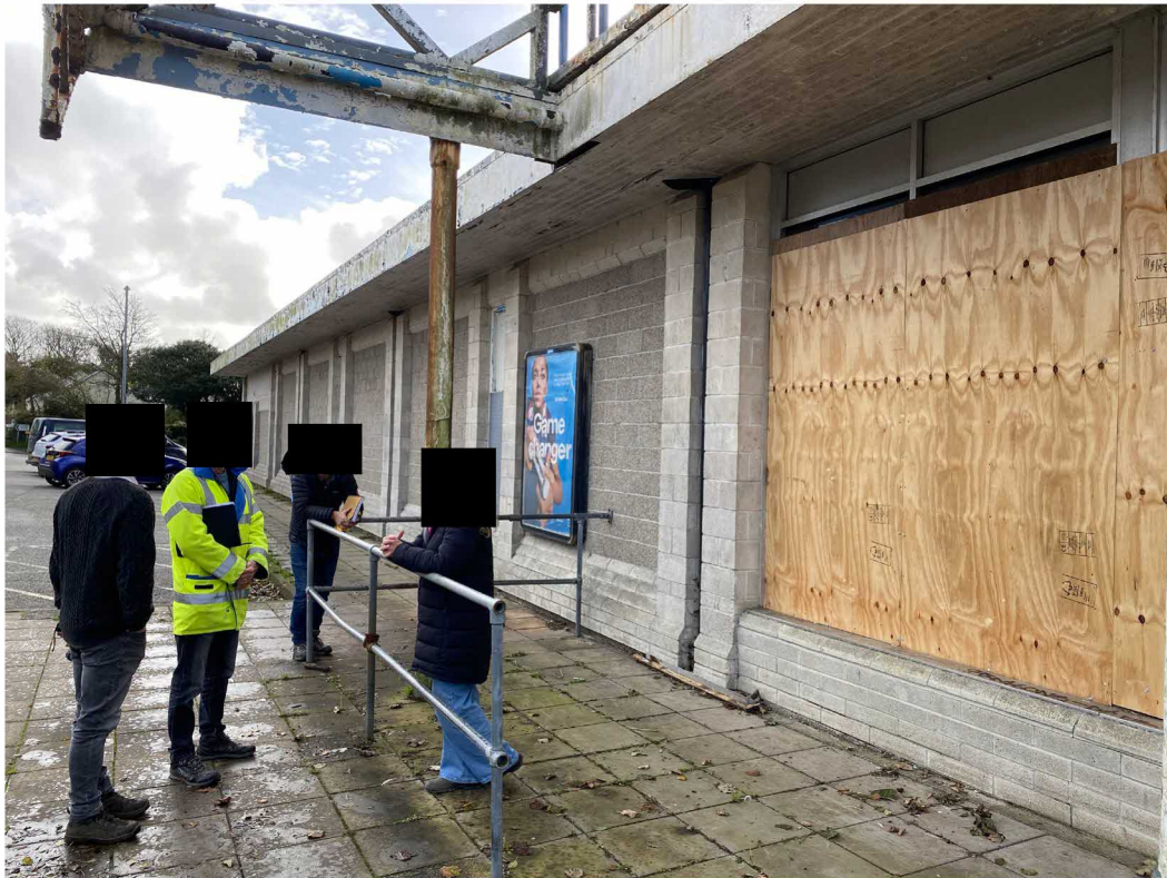
North-East elevation: Boarded up glazing and dilapidated canopy steelwork and railings
