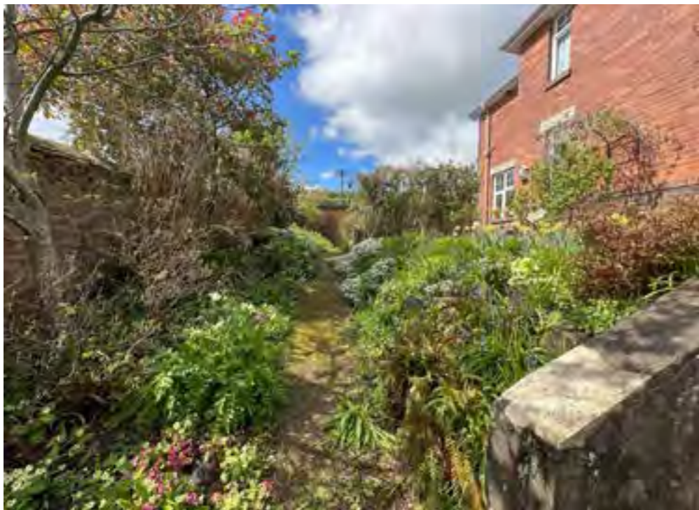
P.5 View along southern elevation with boundary wall to the left of frame.
