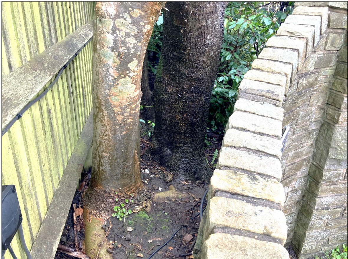
Fig.2 Bases of Ash trees T1 and T2 adjacent to the brick boundary wall, which is cracked.
