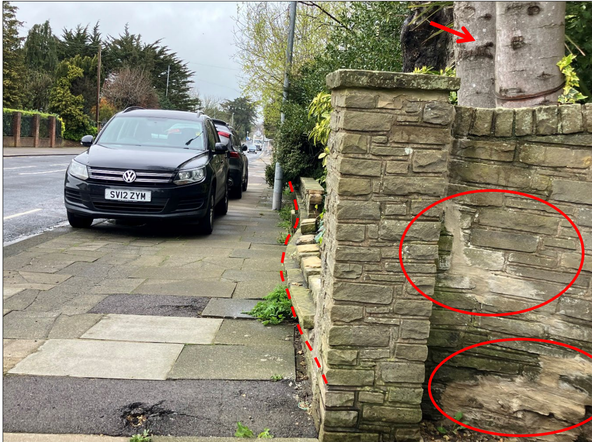
Fig. 4 - Sycamore T3 trunks arrowed and temporary damage repairs in cracked wall. The front boundary wall has now been forced over the public highway, which cannot be resolved where the Sycamore tree is retained.
