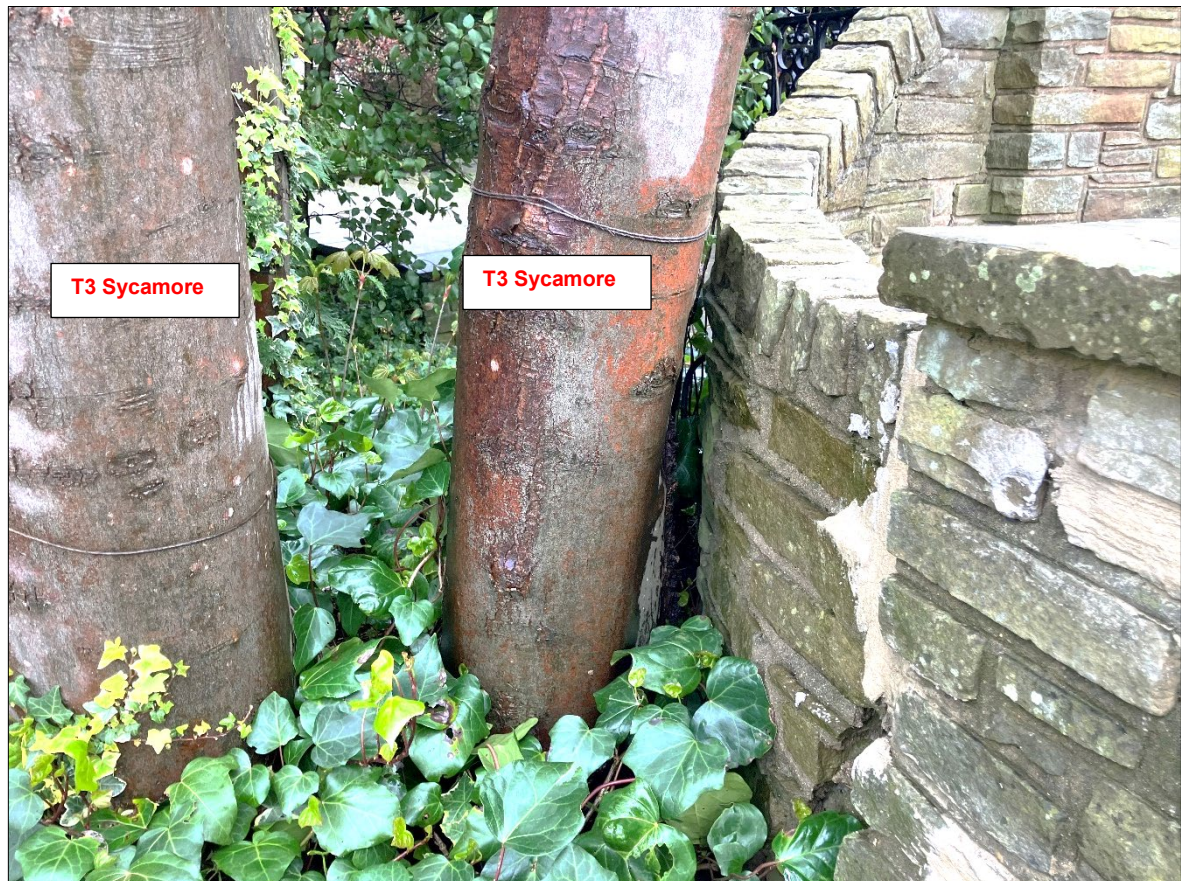
Fig. 3 T3 Sycamore stems adjacent to boundary wall and gate piers, which have been damaged.
