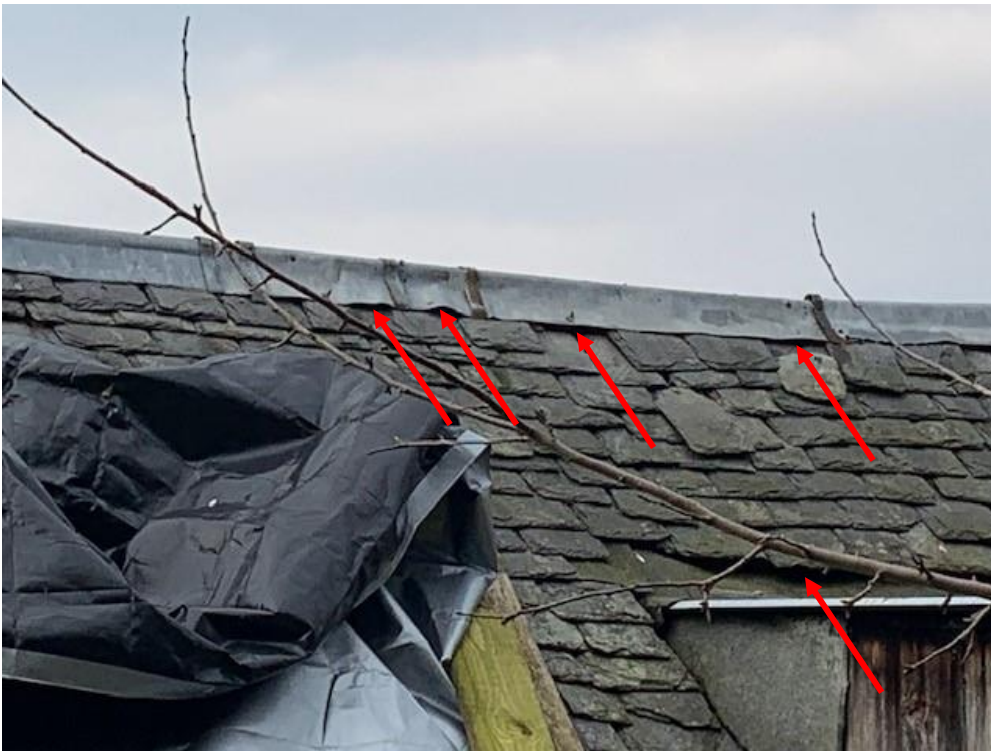
Photo 4. The north side of the garage. Example gaps under ridge flashing and roof slates which provide bat roosting potential are indicated by red arrows.
