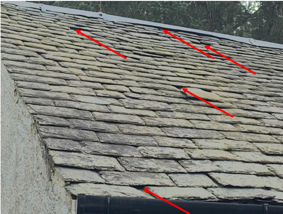
Photo 2. The roof of the south side of the garage with example gaps under roof slates and ridge flashing which provide bat roost potential indicated by red arrows.
