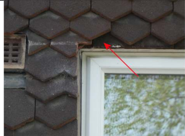
Photograph 32. Opening under hanging tiles at the corner of the window on the east elevation of Nos 7 and 8
