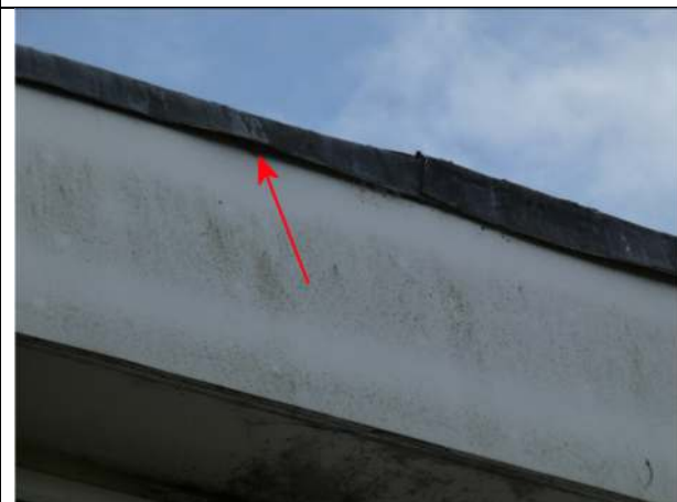
Photograph 47. Opening under the roof edge trim on the east elevation of Nos 13 and 14
