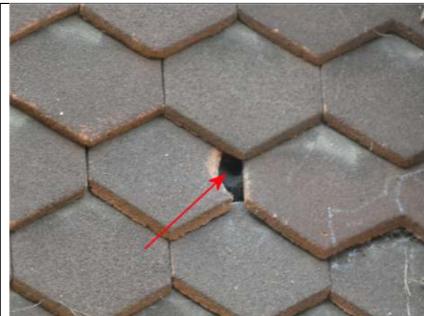
Photograph 17. Opening in the hanging tiles on the east elevation of Nos 3 and 4
