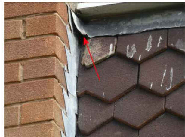
Photograph 41. Opening under lead the roof edge trim under a window on the west elevation of Nos 11 and 12
