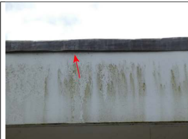
Photograph 9. Lifted roof edge trim on the east side of Nos 1 and 2
