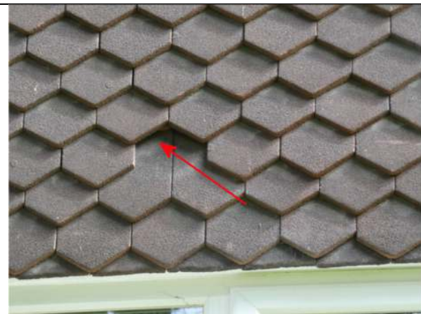
Photograph 22. Missing slate on the west elevation of Nos 5 and 6
