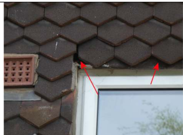
Photograph 48. Opening under hanging tiles above a window on the east elevation of Nos 13 and 14
