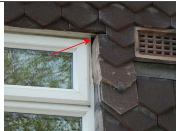
Photograph 33. Opening under hanging tiles at the corner of the window on the east elevation of Nos 7 and 8
