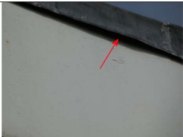
Photograph 10. Lifted roof edge trim on the south side of Nos 1 and 2
