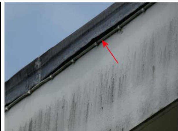
Photograph 11. Lifted roof edge trim on the west side of Nos 1 and 2
