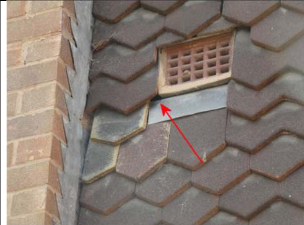
Photograph 19. Opening in the hanging tiles by the vent on the east elevation of Nos 3 and 4
