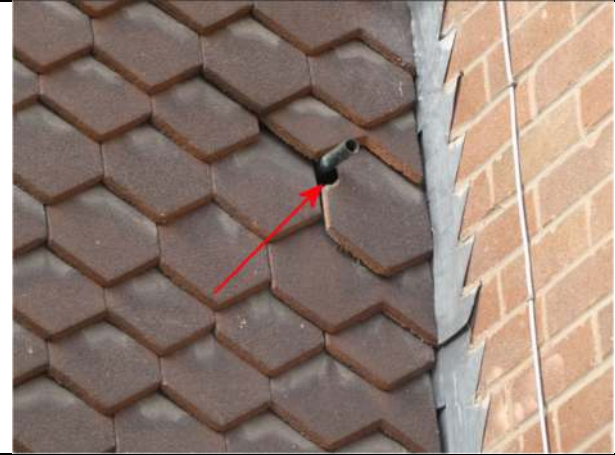
Photograph 26. Opening in the hanging tiles on the east elevation of Nos 5 and 6
