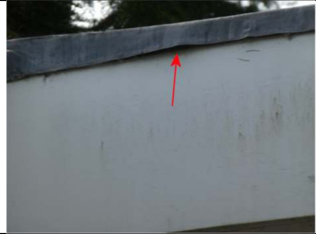
Photograph 38. Opening under the roof edge trim on the east elevation of Nos 9 and 10
