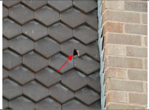
Photograph 8. Hole in a hanging tiles on the east side of Nos 1 and 2
