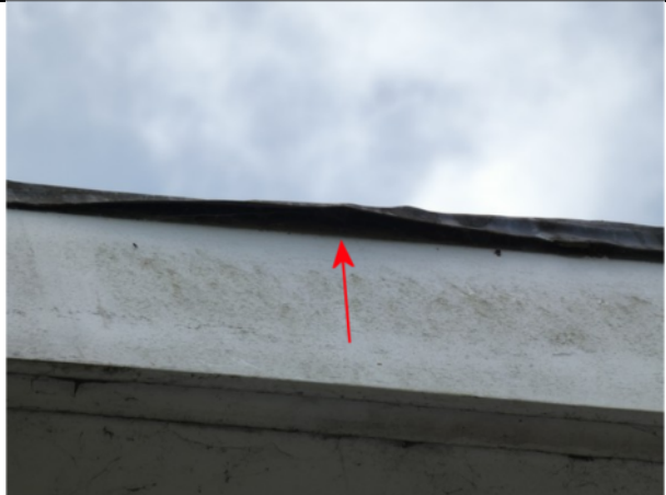
Photograph 50. Opening under the roof edge trim on the east elevation of Nos 13 and 14
