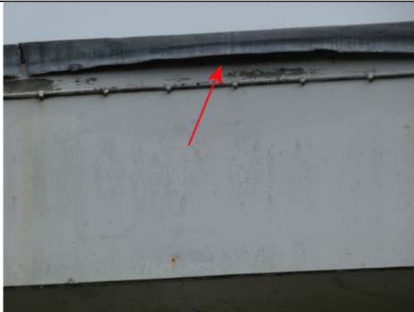
Photograph 51. Opening under the roof edge trim on the east elevation of Nos 13 and 14
