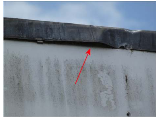
Photograph 15. Opening under the roof edge trim on the east elevation of Nos 3 and 4
