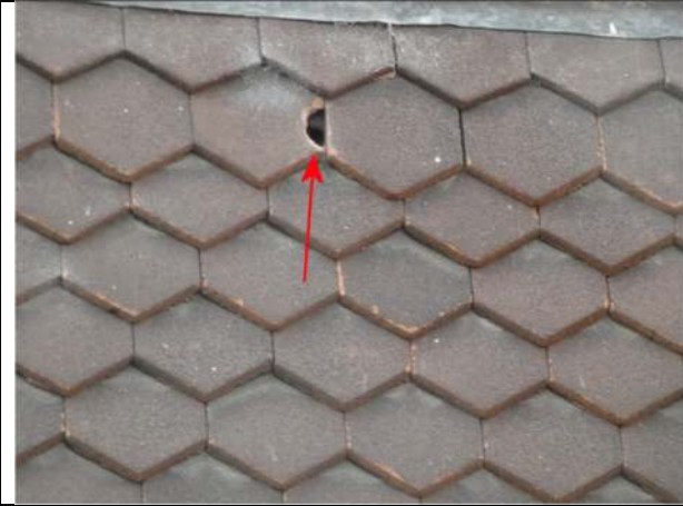
Photograph 43. Opening in the hanging tiles on the east elevation of Nos 11 and 12
