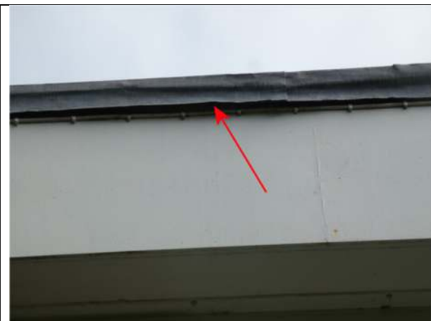
Photograph 23. Opening under the roof edge trim on the west elevation of Nos 5 and 6
