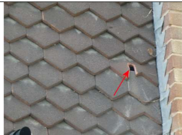
Photograph 34. Opening in the hanging tiles on the east elevation of Nos 7 and 8
