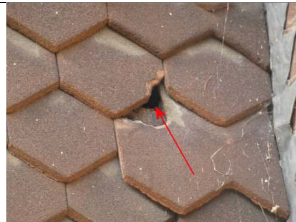
Photograph 18. Opening in the hanging tiles on the east elevation of Nos 3 and 4
