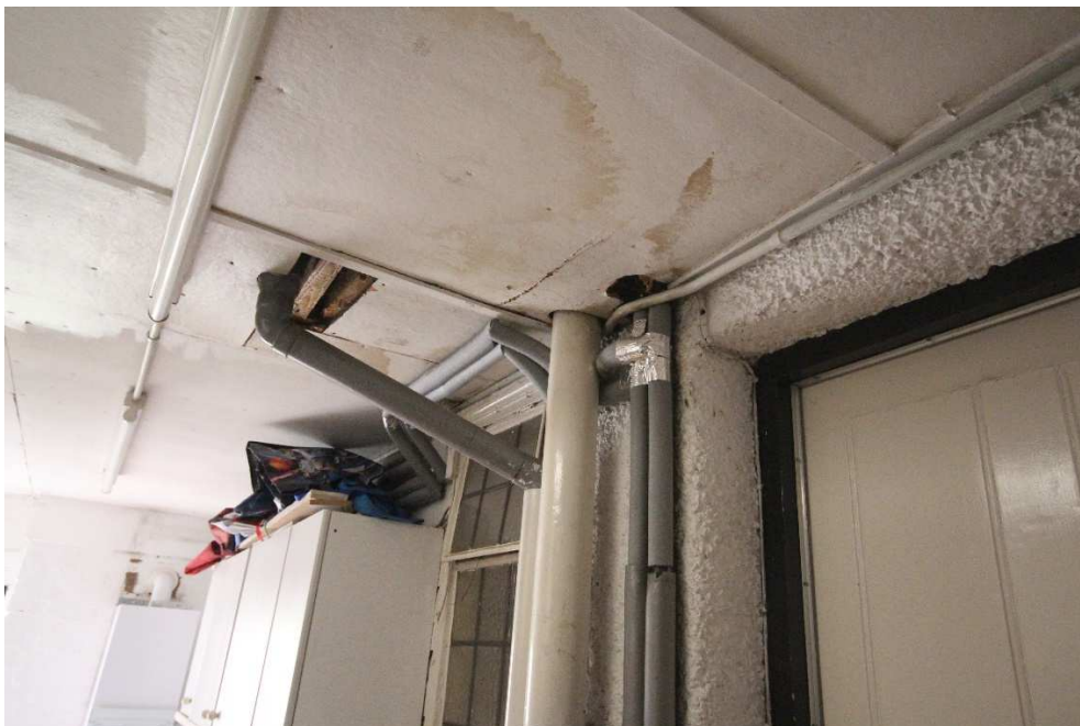
Existing felt roofs to side extensions are in a state of disrepair as evidenced internally
