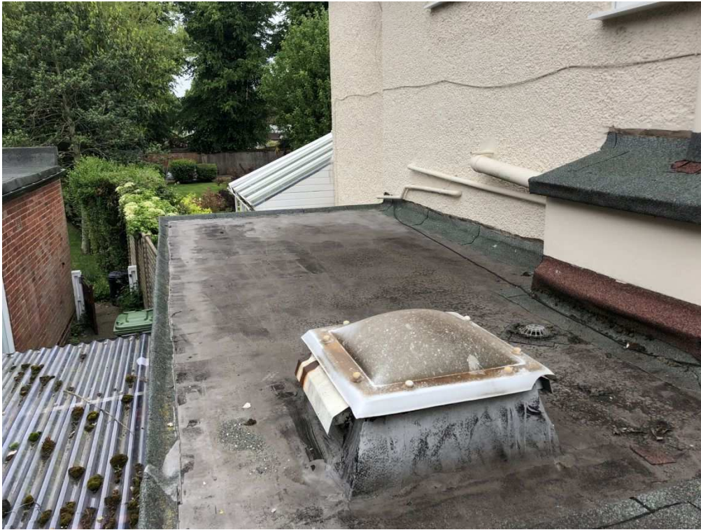
Existing felt roofs to side extensions are in a state of disrepair
