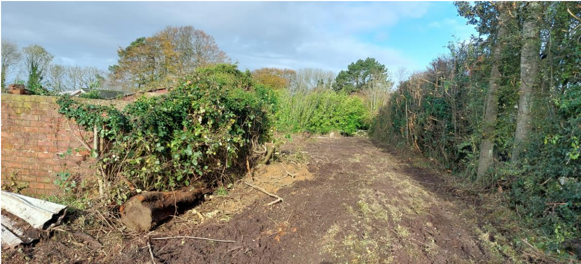
Image 01 – View (south to north) of the artificial unvegetated unsealed surface, with building B02 and a log pile on the left side.
