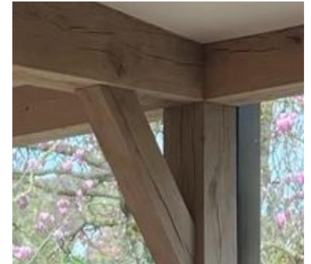
Timber frame externally exposed – Green Oak or similar – left to grey naturally.
