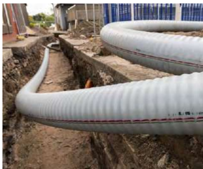
District heating & heat networks
