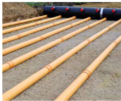
Ground-air heat exchanger
