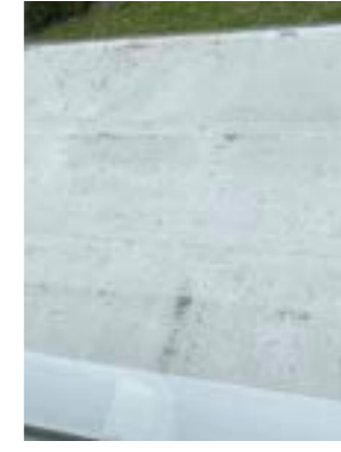
Light grey membrane flat roof
