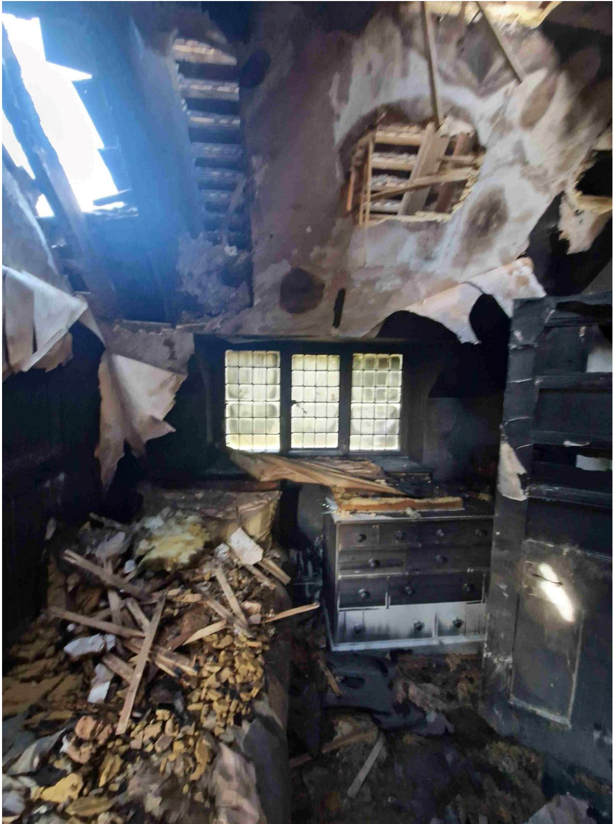
Damaged bedroom 03 (with en suite)
