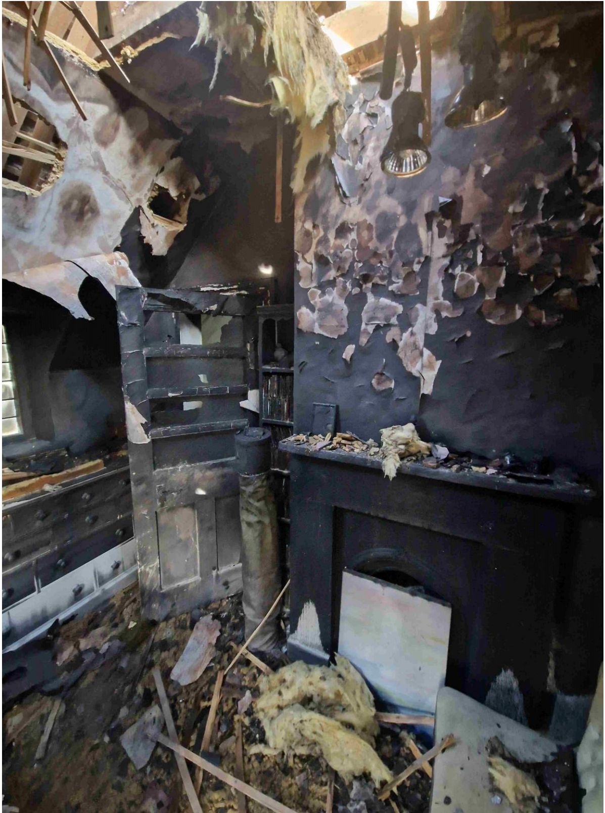
Damaged bedroom 03 (with en suite)
