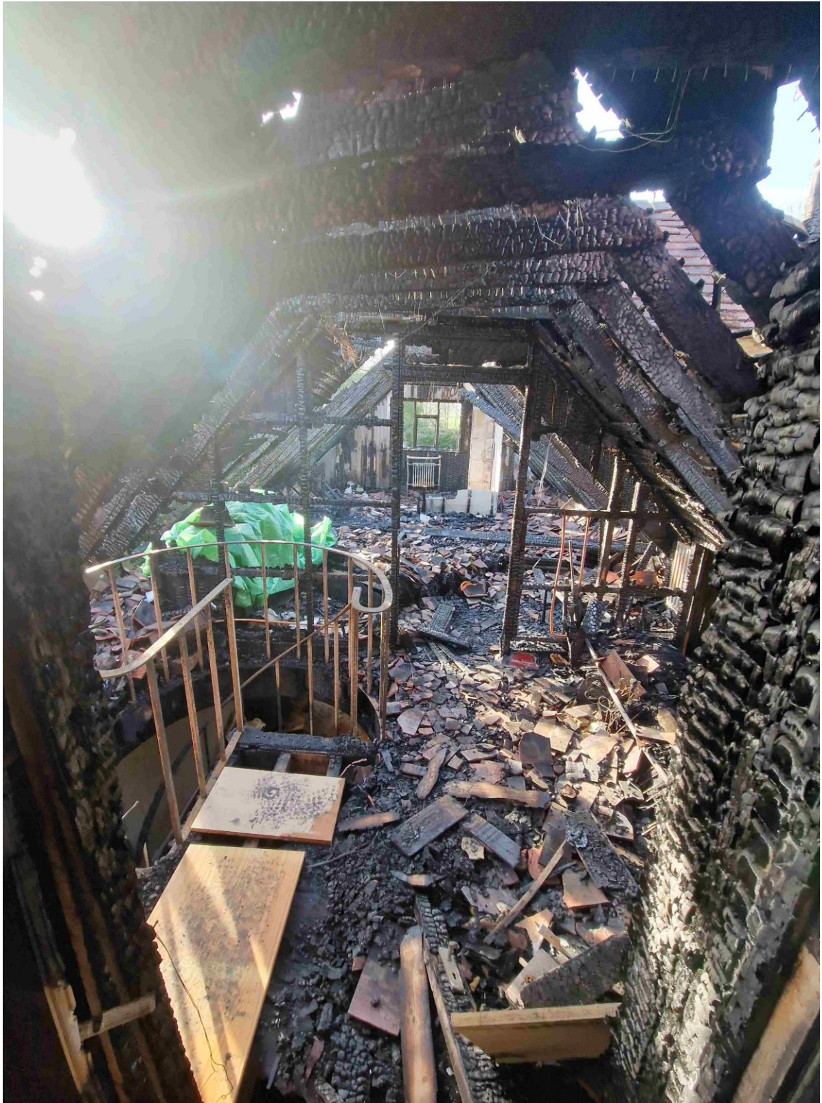
Damaged rooms in Stable section – dressing room, bedroom 04 (rear) and en suite
