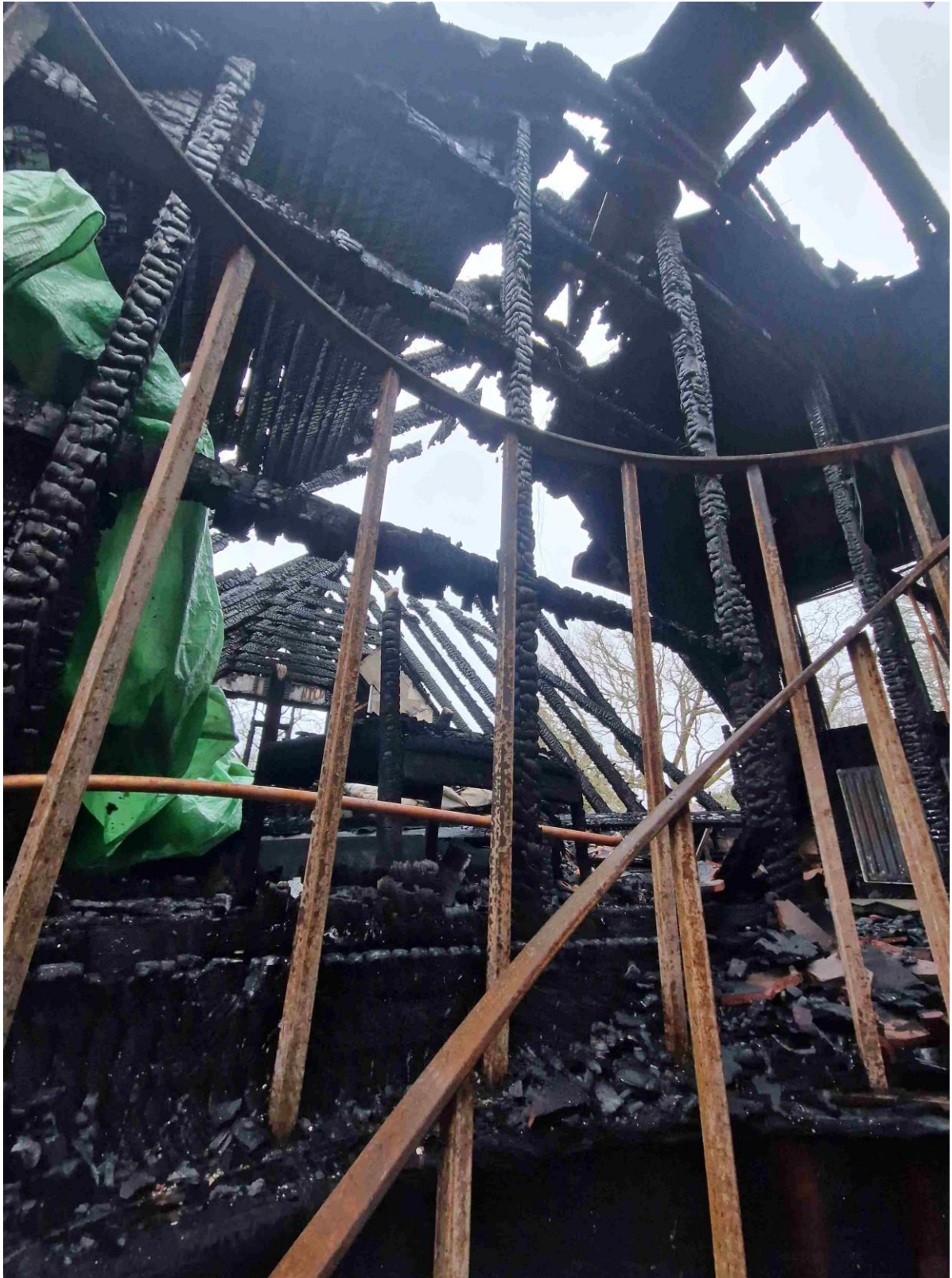
Damaged Stable section
