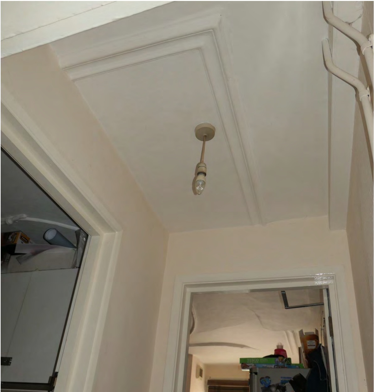
Photo 21: The same ceiling, seen from the lobby to the north of the kitchen.
