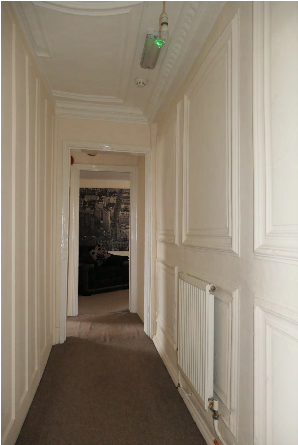
Photo 15: The corridor that has been driven through the central first floor front room (the inserted wall is on the left and the plaster panels on the right).
