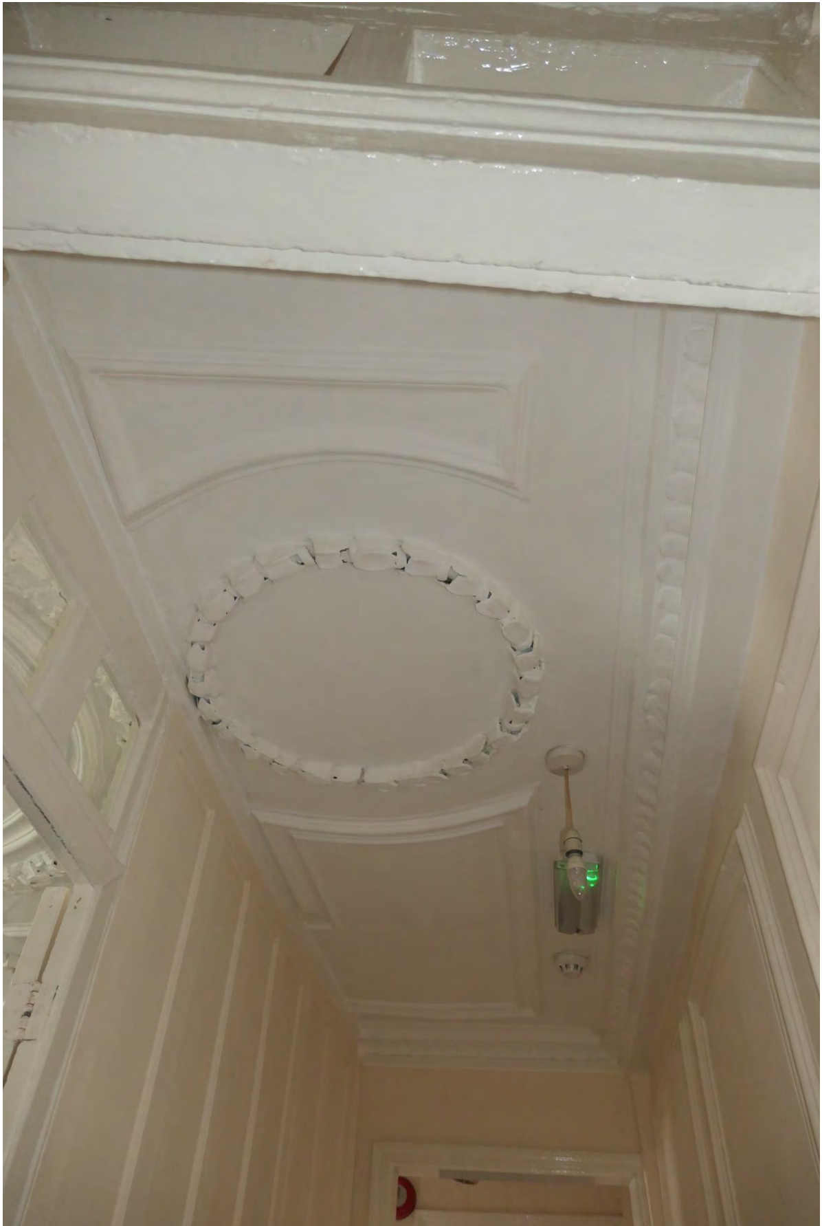
Photo 16: The ceiling where the corridor has been driven through the central first floor front room (the inserted wall is on the left).
