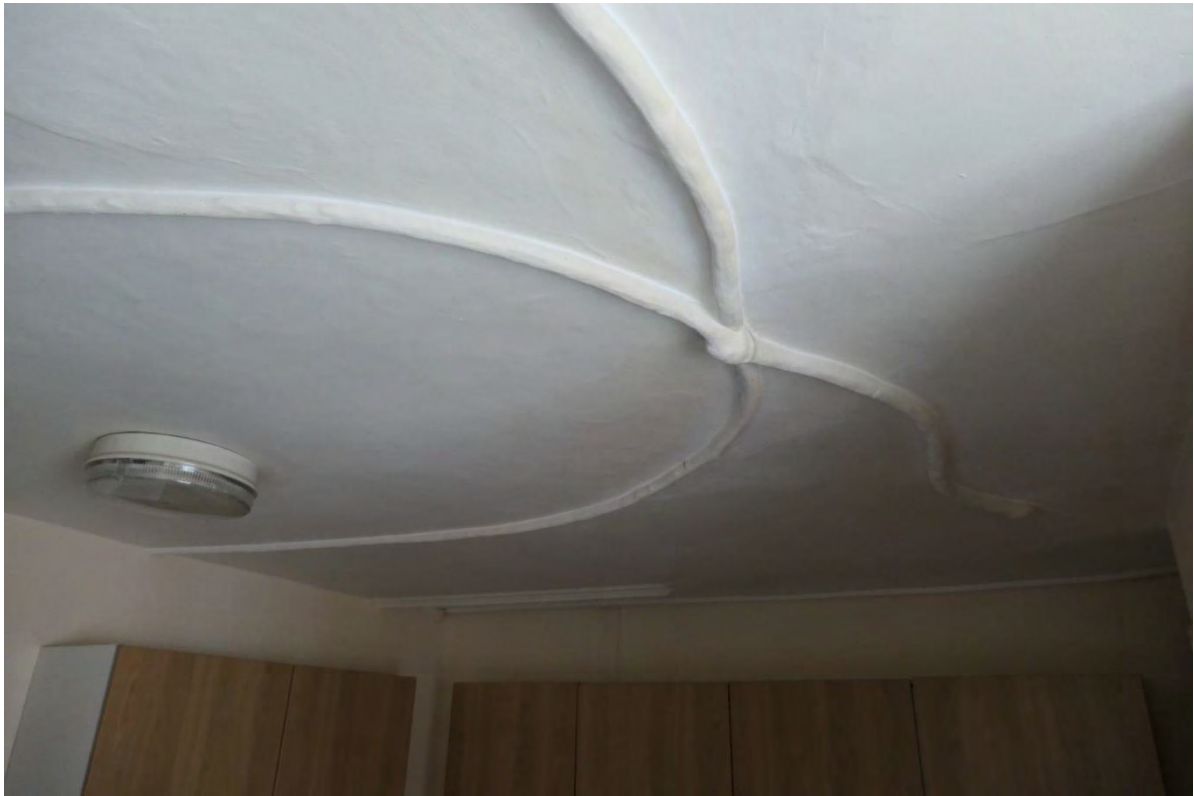
Photo 22: The ceiling in the kitchen area centrally at the rear of the first floor.
