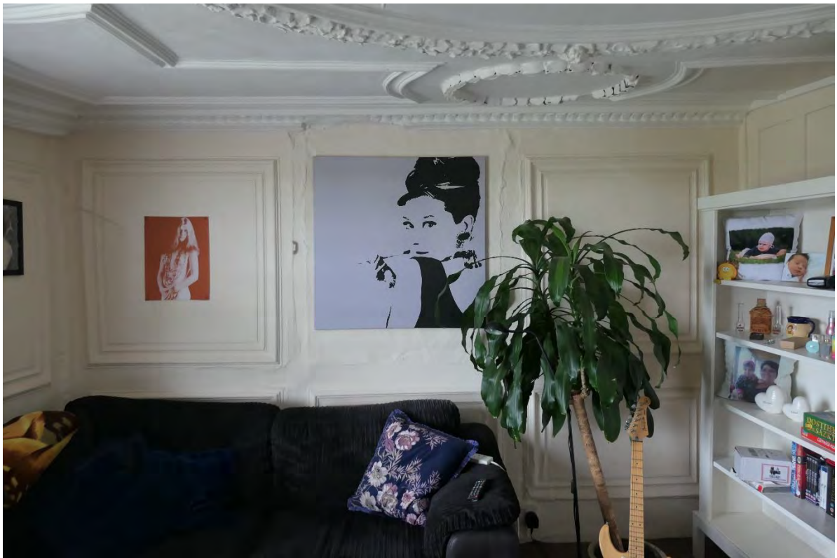
Photo 18: The east wall with missing plaster panel in the central first floor front room.
