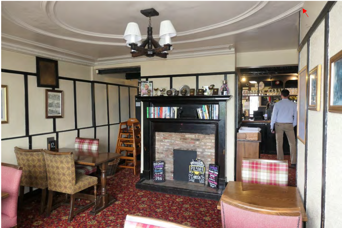
Photo 8: The NE ground floor room. the red arrow on the right shows where the plaster ceiling has been truncated by the stairwell.
