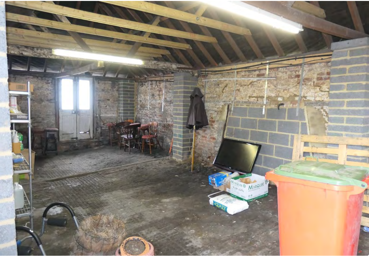
Photo 27: Internally the building has been substantially rebuilt and it is devoid of any features of note.
