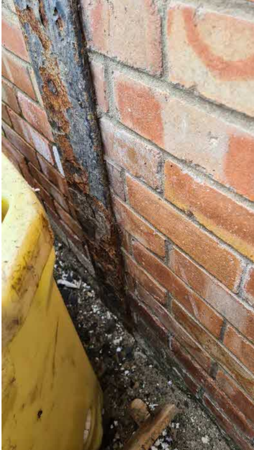
Figure General Image Showing the Storage of Materials/Equipment I Beam Severe corrosion / delamination
