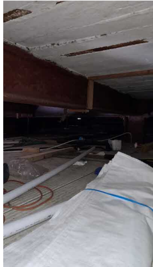
Figure Jacks Place Internal Support structure above holding tanks
