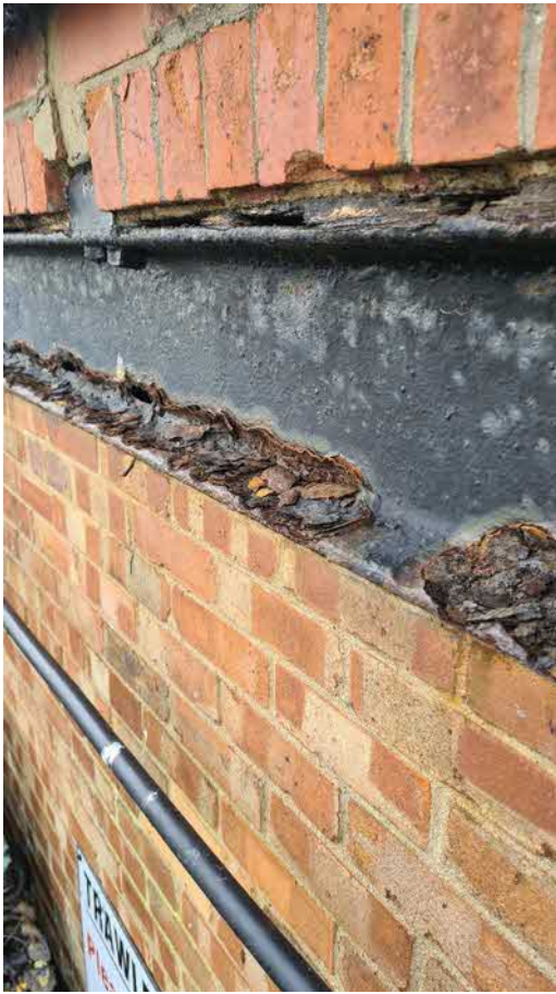
Figure Location 4 I Beam Severe corrosion / delamination
