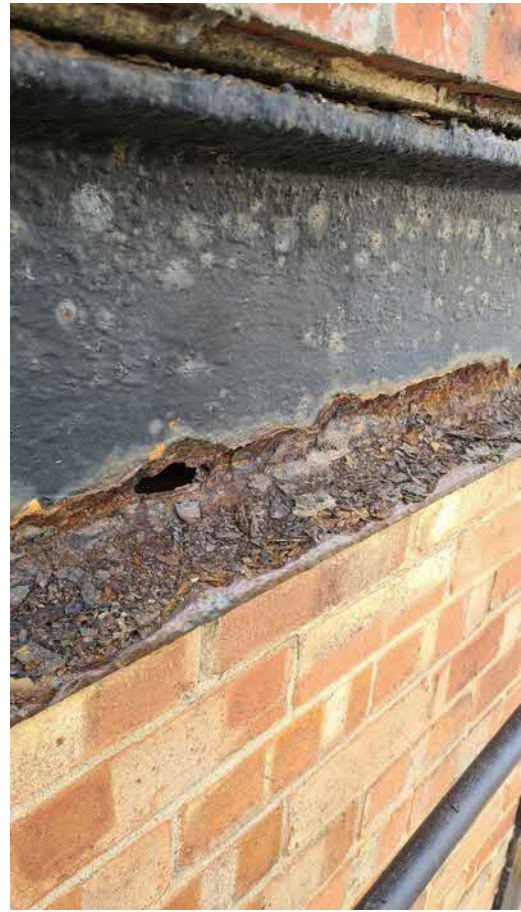
Figure Location 4 I Beam Severe corrosion / delamination
