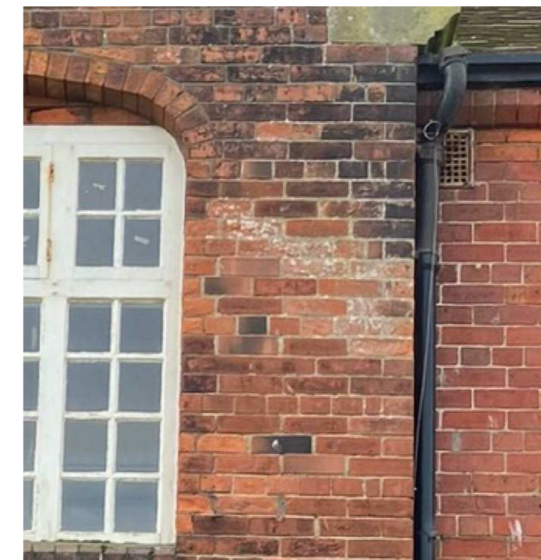
Example area of Masonry condition requiring cleaning
