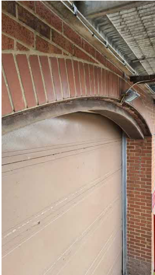
Figure Steel Lintel distortion & flashing separation
