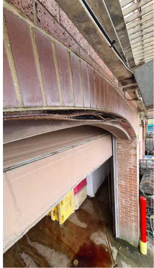
Figure Steel Lintel distortion & flashing separation
