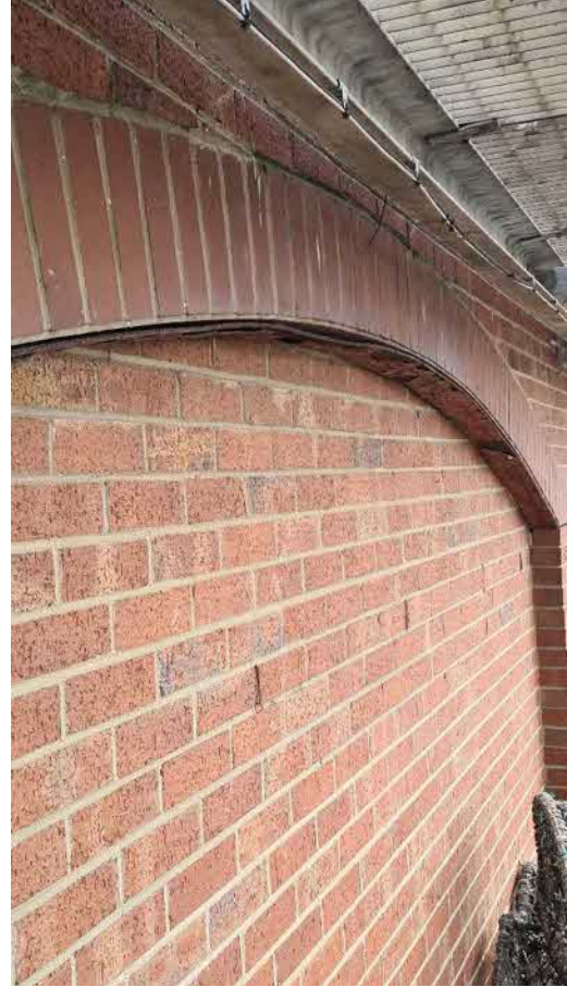
Figure Steel Lintel distortion & flashing separation
