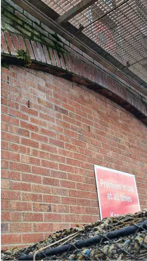
Figure Steel Lintel distortion & flashing separation
