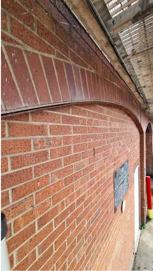
Figure Steel Lintel distortion
