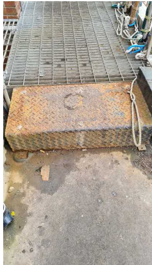
Figure Front gantry step from building 2 – 3 is loose
