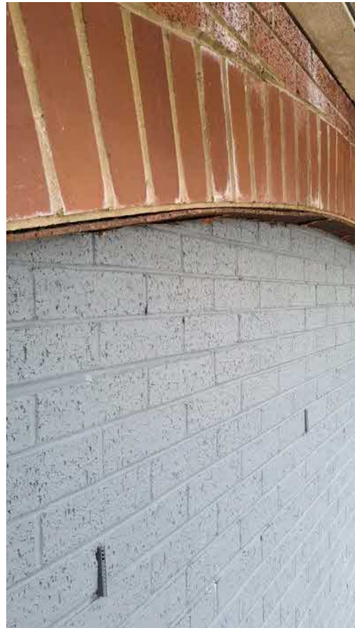
Figure Steel Lintel distortion
