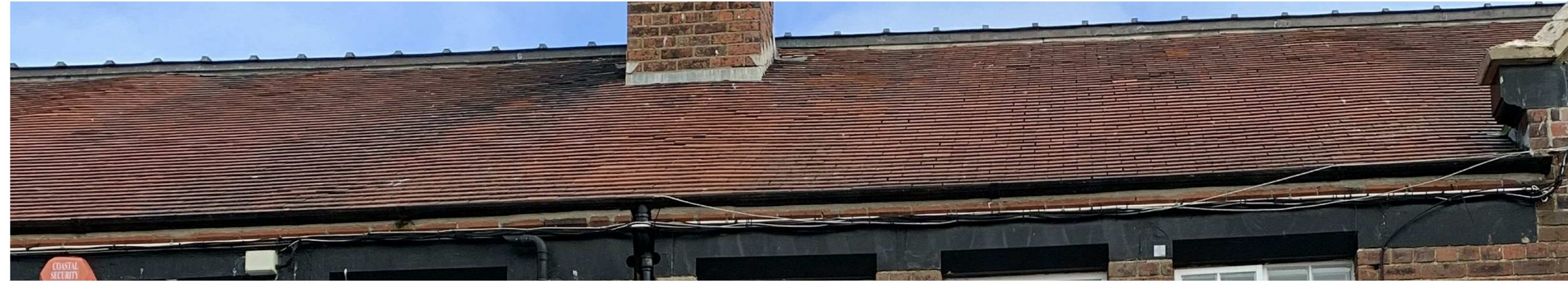
Example of requirement to repair Roof Structure, and condition of Roof Tiles (Also note Cast Iron Rainwater Goods, and Brick specials to underside)
