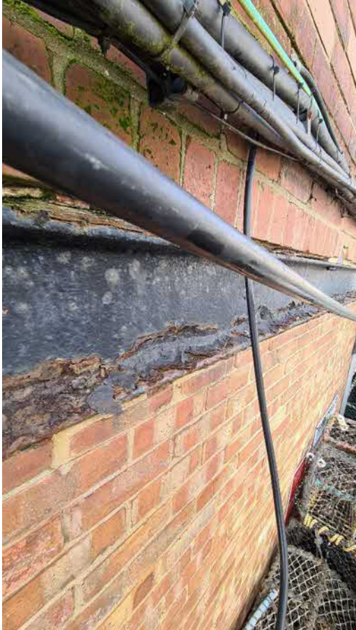
Figure Location 5 I Beam Severe corrosion / delamination
