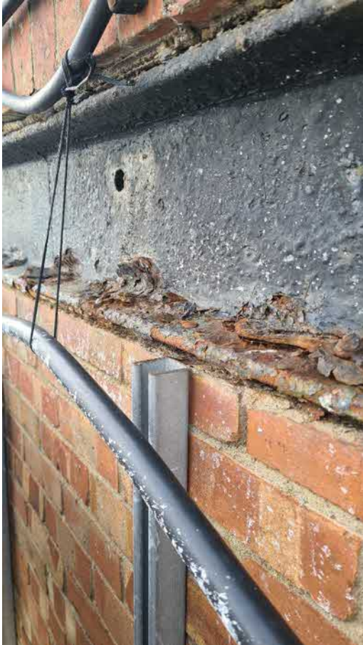
Figure General Image I Beam Severe corrosion / delamination
