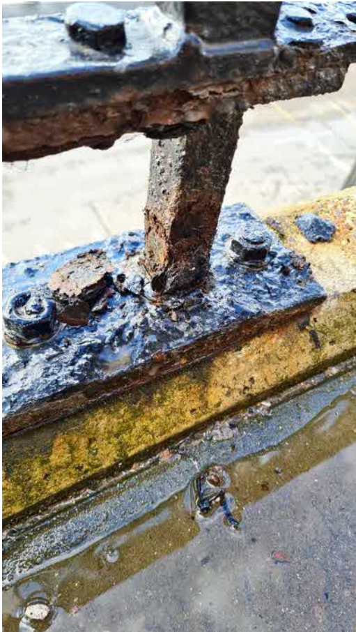
Figure Balcony Handrail, severe corrosion
