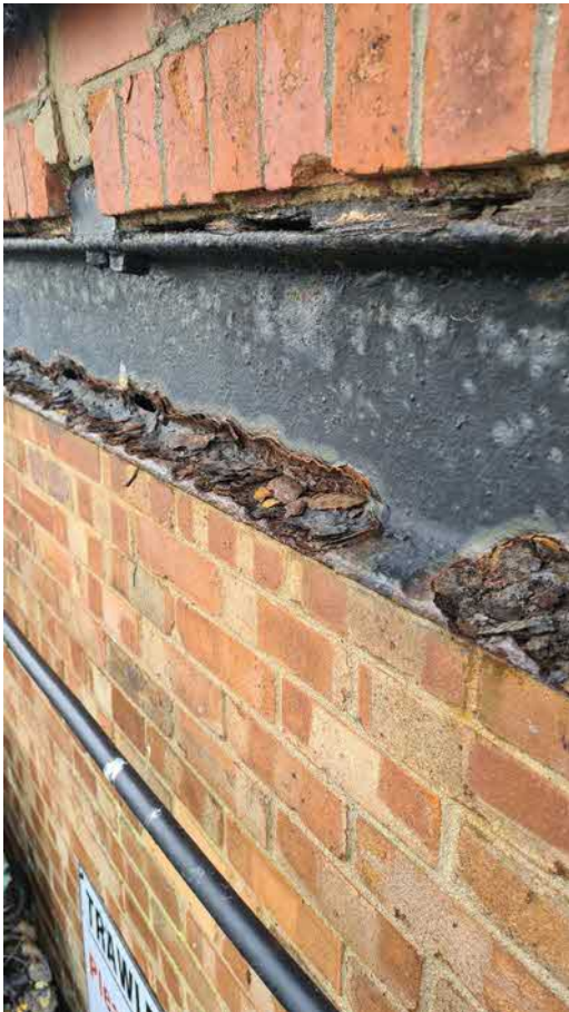
Figure Location 4 I Beam Severe corrosion / delamination
