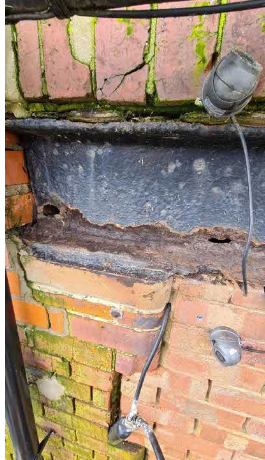
Figure Location 5 I Beam Severe corrosion / delamination
