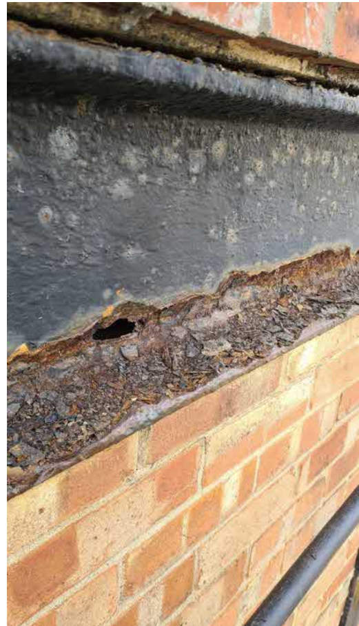
Figure Location 4 I Beam Severe corrosion / delamination
