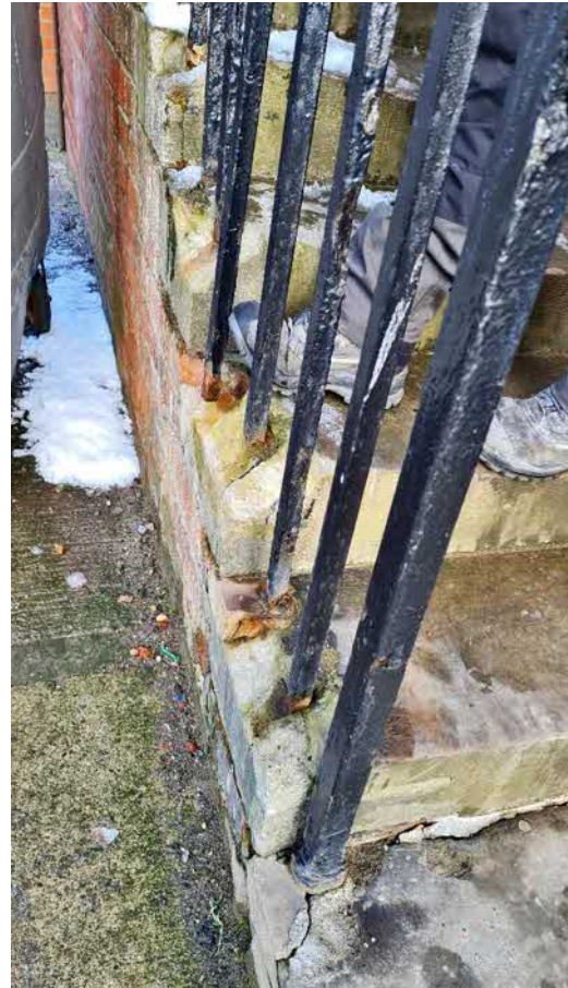
Figure Failed Stanchions Handrail severe corrosion. Spalling concrete
